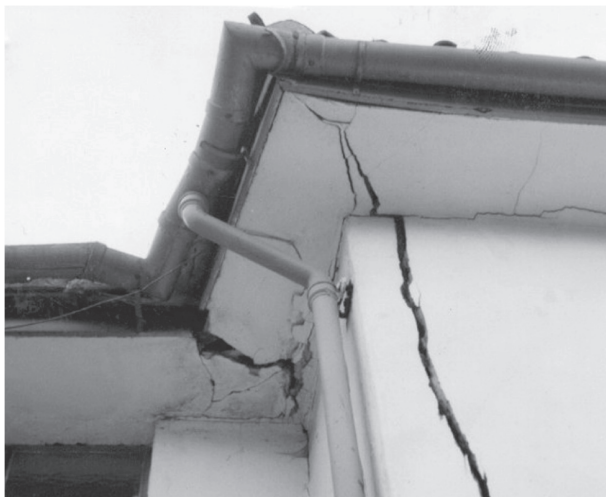
Figure 33.1 Structural damage to house caused by ‘end lift’ © Peter Kelsey & Partners
