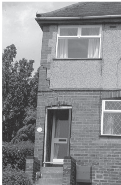
Figure 33.2 Example of differential settlement due to influence of trees
