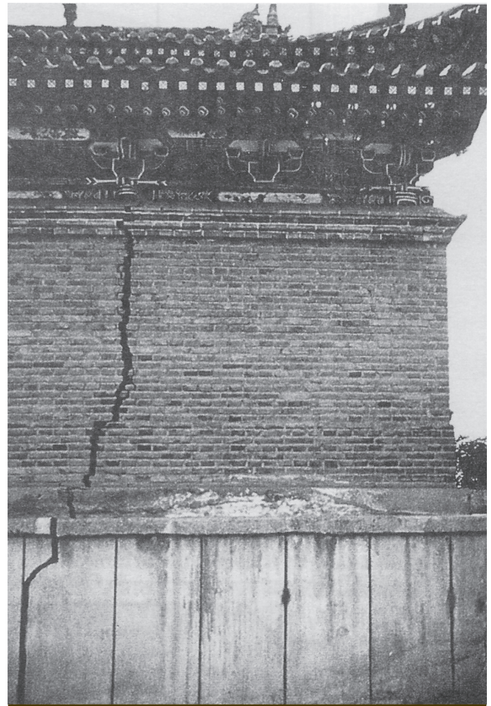
Figure 32.3 Collapse-induced cracking in a 15th century pagoda Reproduced from Billard et al. (2000); John Wiley & Sons, Inc.
