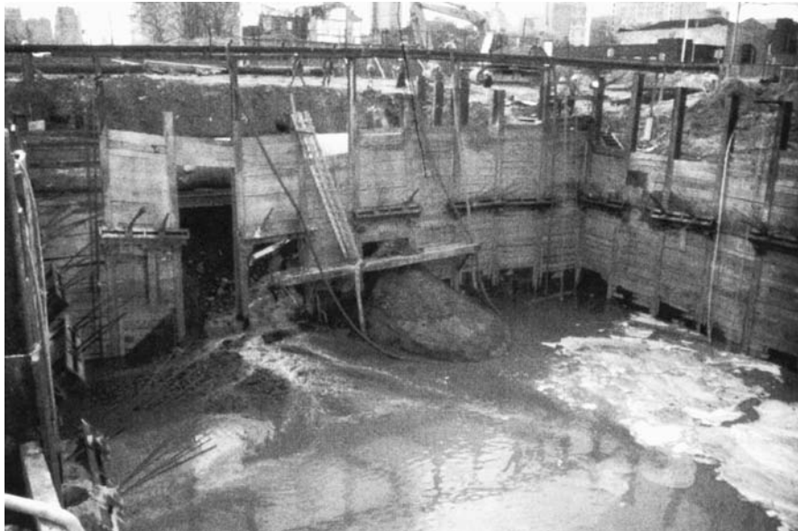
FIGURE 14.1 Damage to a braced excavation by seepage forces. (Courtesy of George Tamaro, Mueser Rutledge Consulting Engineers.)
