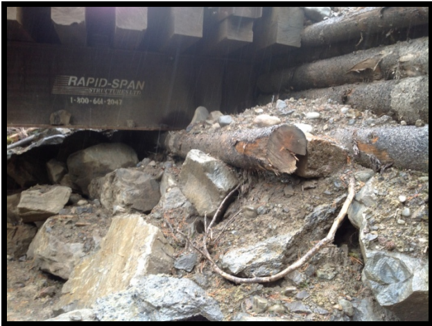
Undersized and improperly located sill log does not adequately support superstructure. Girder stiffener and bearing plate does not align with center of sill
