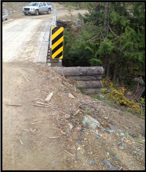
No approach logs or approach flares to direct traffic onto bridge deck prevent vehicles from dropping off road prism edge.
