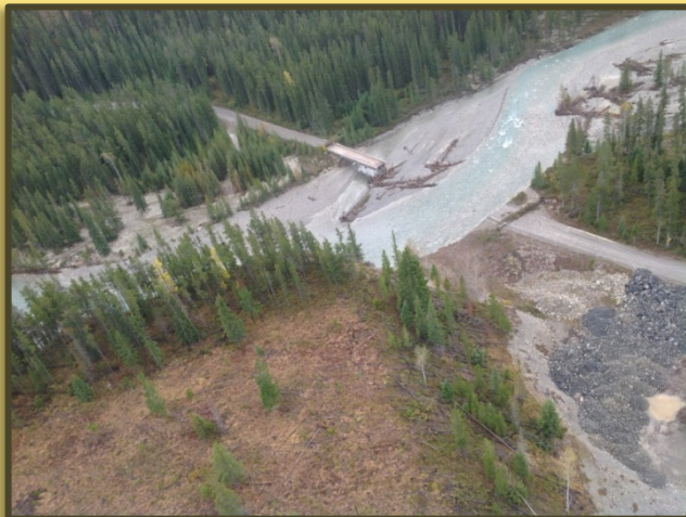
FSR bridge over the White River destroyed by June storm event.
