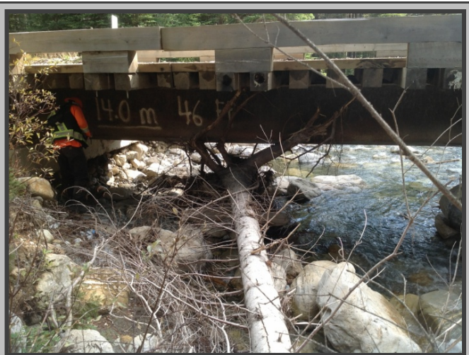
Inadequate clearance. Debris is trapped under bridge.
