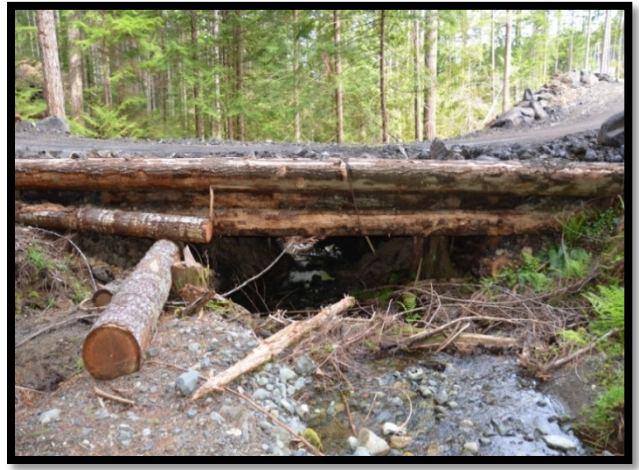
Bridge located at the bottom of a hill, on a curve and there are no guard rails. Superstructure was not lashed or pinned properly to the foundations. No consideration for unbalanced loads or off-centre driving. This bridge was examined during a 2013 audit.
