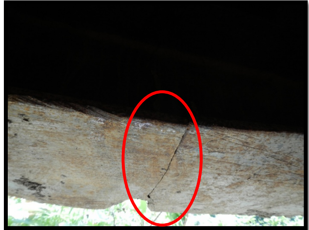
Crack in underside of I-beam of portable bridge. Expanded under live load.
