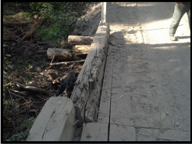
Deck panels differ in width. Narrow panel shows damage from a vehicle.
