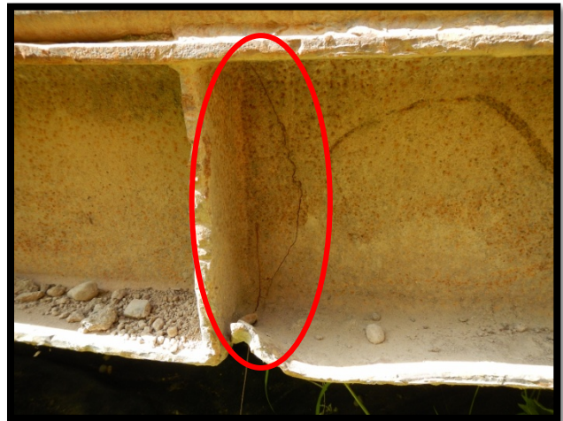
Same portable bridge indicating I beam fatigue that expanded under live load.
