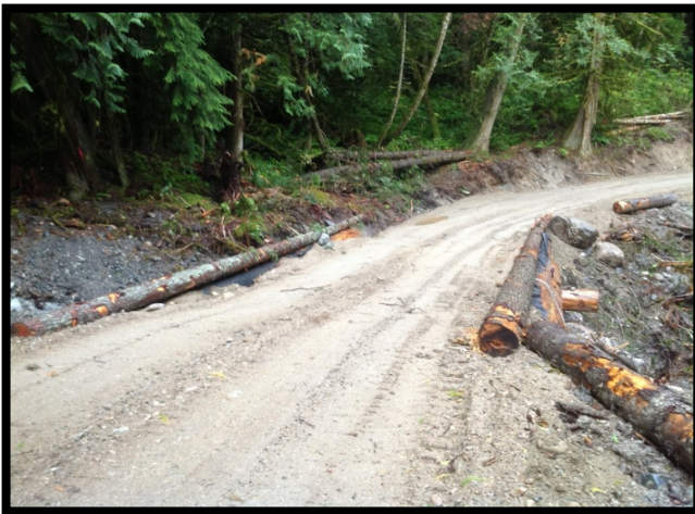
These curb logs are not attached to the bridge and are ineffective if struck by a vehicle. Potential for a vehicle to accidentally drive off the bridge.
