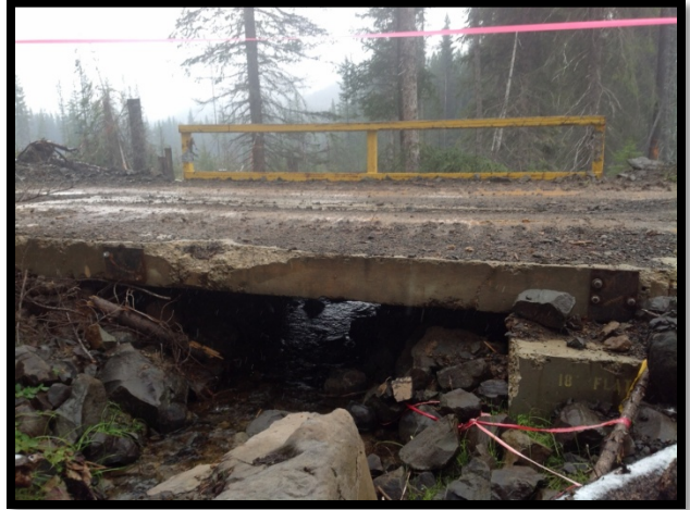
Concrete slab bridge missing guard rail.
