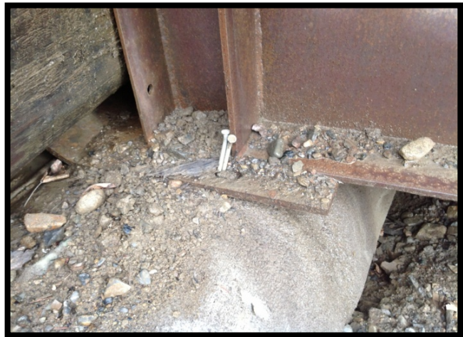
Superstructure attached improperly to round sill and bearing plate is not fully supported and aligned on the sill.
