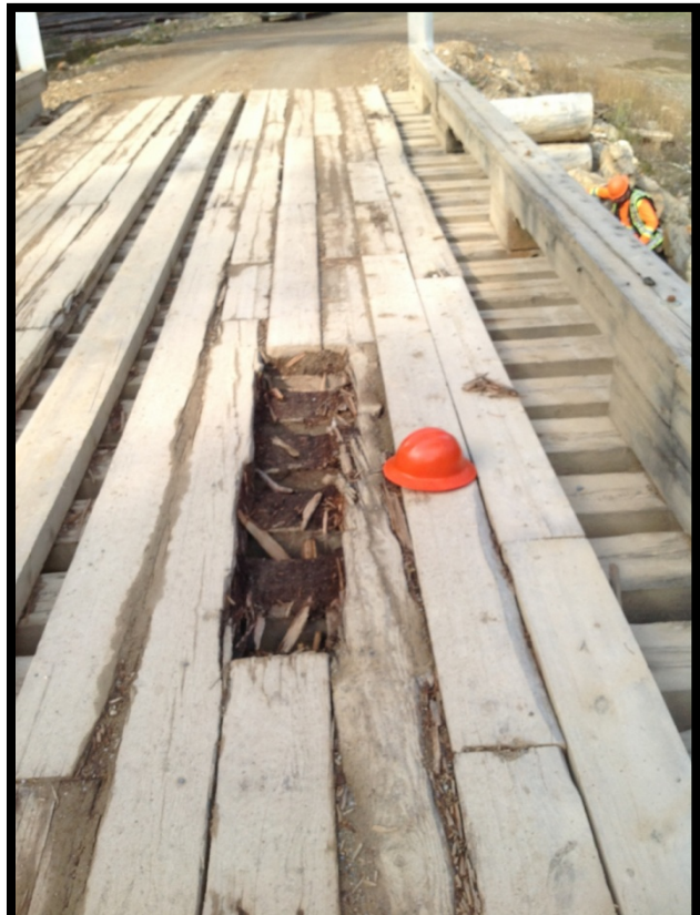
Deck rotten/ damaged and a significant gap between running surface and the guard rail could catch a wheel.
