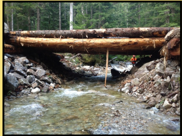
This bridge is too short for the stream and the rip-rap is constricting the channel. Natural surface drainage is not maintained.
