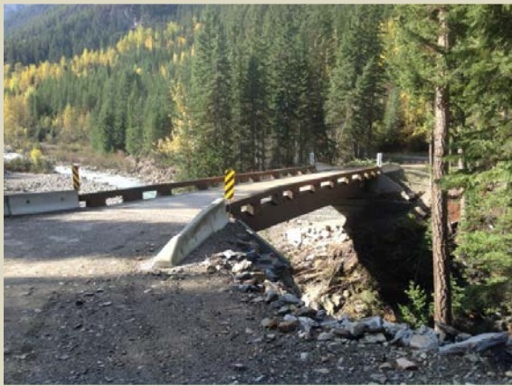
This bridge has concrete "no-posts" on the approaches to direct traffic onto the bridge deck.
