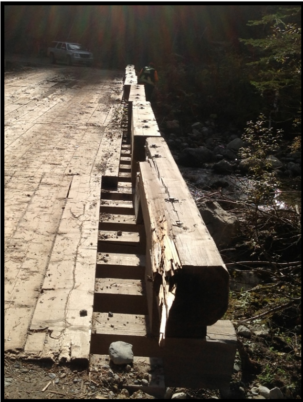
Deck panels have shifted because they are not attached to the girders.
