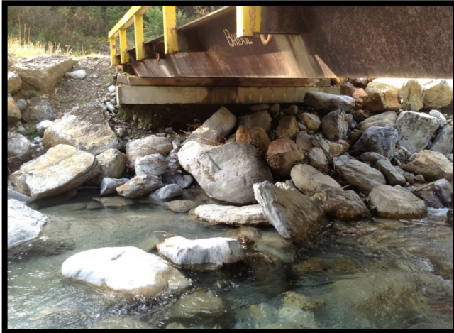
Abutment erosion resulting from inadequate foundations installed well above creek scour depth, constructed within stream channel. An improperly supported substructure could ultimately result in structural failure of the bridge.
