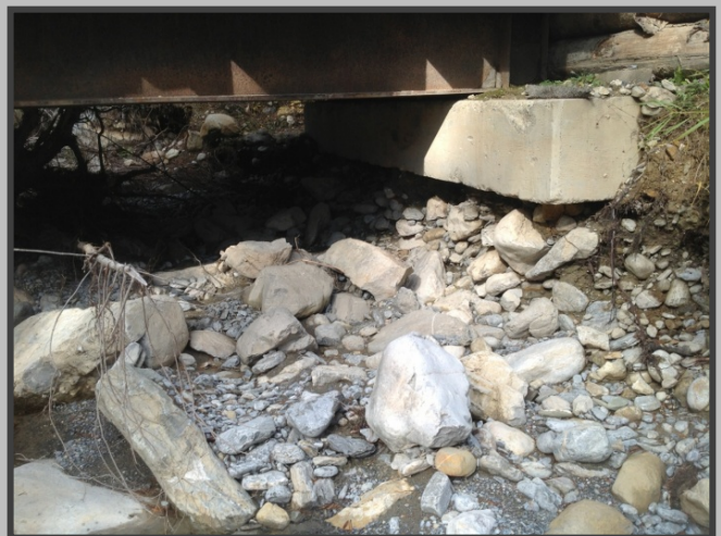
Erosion of the sill on the same bridge due to inadequate clearance.
