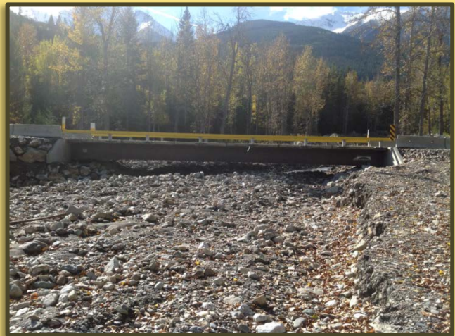
Insufficient clearance after a storm event due to aggradation (deposited sediment and gravel).
