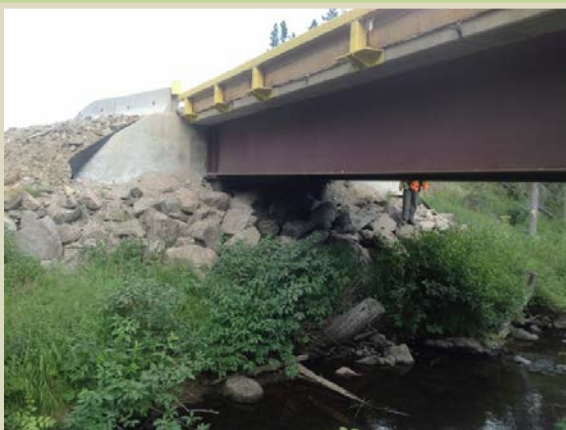
This bridge abutment is well armored and placed outside of the stream channel to prevent scour.
