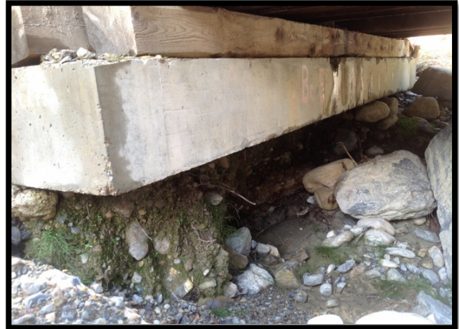
Close-up of same bridge. Extensive scour under the foundation after a major storm event.
