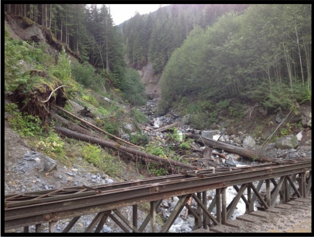
Unstable channel above bridge with no consideration of channel geomorphology or anticipated flows. No information provided by licensee.
