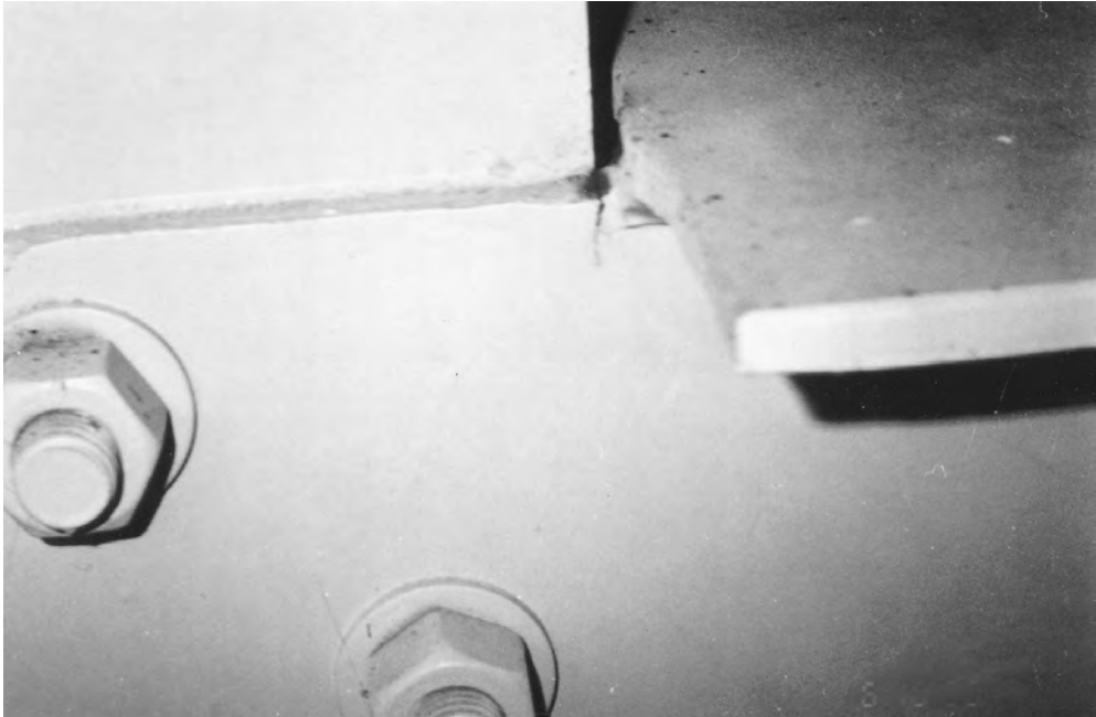
FIGURE 53.8 Close-up view of a crack originating at the termination of a flange on a floor beam with a “simple” connection to an attachment plate in the Dresbach Bridge in Minnesota. The crack is an indication of an end moment in the simple connection that is not predicted in design.
