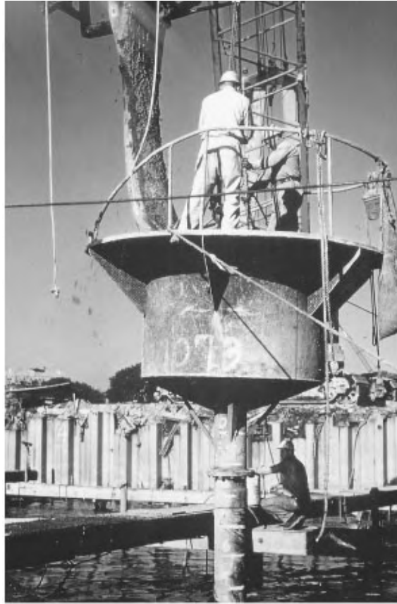
FIGURE 47.14 Placing underwater concrete through hopper and tremie pipe, Verrazano Narrows Bridge, New York.
