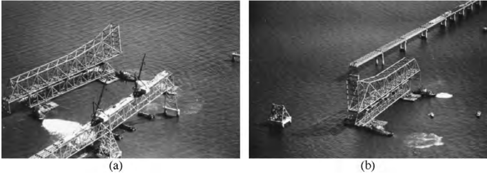
Figure 45.30 Floating-in erection of a truss span, first Chesapeake Bay Bridge, Maryland, 1951. Erected 300 ft (91 m) deck-truss spans form erection dock, providing a work platform for two derrick travelers. A permanent deck-truss span serves as a falsework truss supported on barges and is shown carrying the 470 ft (143 m) anchor arm of the through-cantilever truss. This span is floated to its permanent position, then landed onto its piers by ballasting the barges. (a) Float leaves erection dock, and (b) float arrives at permanent position. (Courtesy of Bethlehem Steel Corporation.)
