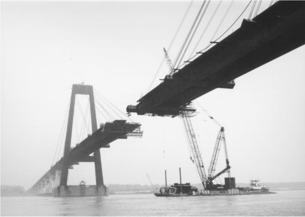
Figure 45.9 Cable-stayed orthotropic-steel-deck bridge over Mississippi River at Luling, La., 1982; view looking northeast. The main span is 1222 ft (372 m); the A-frame towers are 350 ft (107 m) high. A barge-mounted ringer derrick erected the main steelwork, using a 340 ft (104 m) boom with a 120 ft (37 m) jib to erect tower components weighing up to 183 tons, and using a shorter boom for deck components. Cable stays at the ends of projecting cross girders are permanent; others are temporary erection stays. Girder section 16-west of north portion of bridge, erected a few days previously, is projecting at left; companion girder section 16-east is on barge ready for erection (see Figure 45.10 ).
