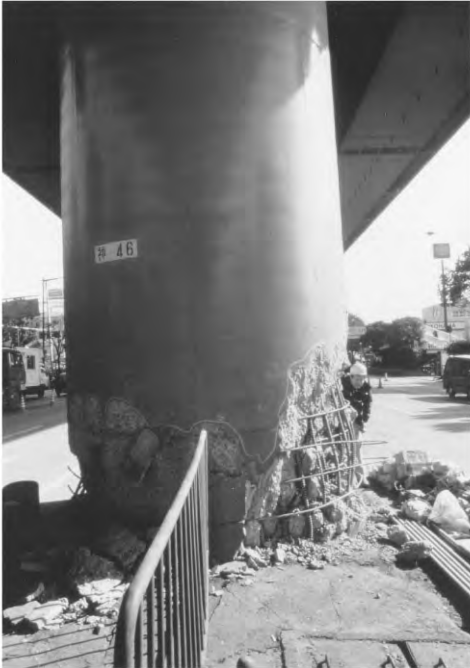
FIGURE 34.18 Hanshin Expressway, Pier 46, damage in the 1995 Hyogo-Ken Nanbu earthquake.
