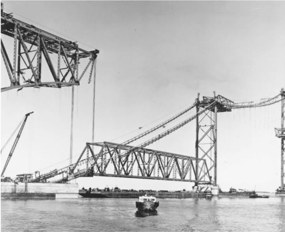
Figure 45.32 Erection of a truss span by hoisting, first Chesapeake Bay Bridge, Maryland, 1952. A 360 ft (110 m) truss span is floated into position on barges and picked clear using four sets of lifting falls. Suspension bridge deck is under construction at right. (Courtesy of Bethlehem Steel Corporation.)
