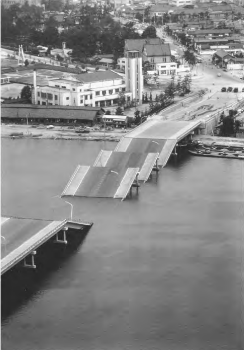
FIGURE 34.8 Showa Bridge collapse in 1964 Niigata earthquake.
