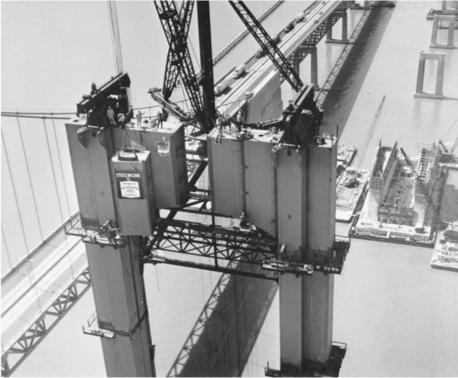
Figure 45.35 Tower erection, second Delaware Memorial Bridge, Wilmington, Del., 1966. The tower erection traveler has reached the topmost erecting position and swings into place the 23 ton closing top-strut section. The tower legs were jacked apart about 2 in (50 mm) to provide entering clearance. The traveler jumping beams are in the topmost working position, above the cable saddles. The tower steelwork is about 418 ft (127 m) high. Cable anchorage pier is under construction at right. First Delaware Memorial Bridge (1951) is at left. The main span of both bridges is 2150 ft (655 m). (Courtesy of Bethlehem Steel Corporation.)
