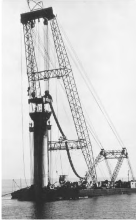
FIGURE 47.8 Installing concrete cylinder pile by internal excavation, jetting, and pull-down force from barge.
