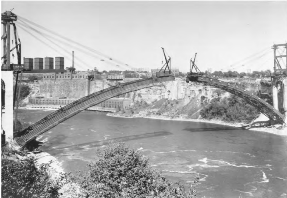
Figure 45.2 Erection of arch ribs, Rainbow Bridge, Niagara Falls, New York, 1941. Bridge span is 950 ft (290 m), with rise of 150 ft 46 m); box ribs are 3 × 12 ft (0.91 × 3.66 m). Tiebacks were attached starting at the end of the third tier and jumped forward as erection progressed (see Figure 45.3). Much permanent steelwork was used in tieback bents. Derricks on approaches load steelwork onto material cars that travel up arch ribs. Travelers are shown erecting last full-length arch-rib sections, leaving only the short, closing crown sections to be erected. Canada is at right, the U.S. at left. (Courtesy of Bethlehem Steel Corporation.)
