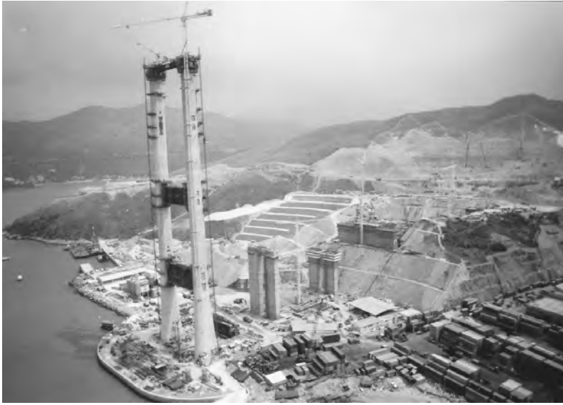
FIGURE 18.27 Tower erection for the Tsing Ma Bridge. (Courtesy of Mitsui Engineering & Shipbuilding Co., Ltd.)
