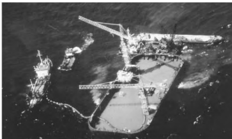
FIGURE 47.27 Prefabricated box caisson is floated into position, Great Belt Eastern Bridge, Denmark. Note temporary cofferdam above concrete caisson.
