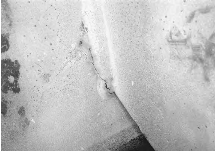
FIGURE 53.6 View of crack in the fillet weld joining the diaphragm connection plate to the web of a box section in the Washington Metro elevated structures. The crack is caused by distortion in the small gap between the bottom of the attachment plate and the box girder flange.
