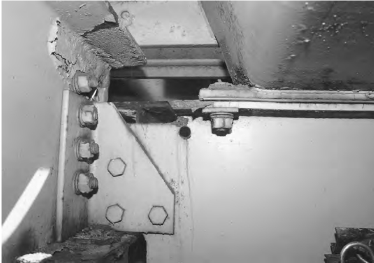
FIGURE 53.5 View of floor beam of Throgg's Neck Bridge in New York showing crack in the cope that has been repaired by drilling a stop hole. The crack is caused by incompatibility between the curvature of the superstructure and the orthotropic steel deck that is bolted onto the floor beams.
