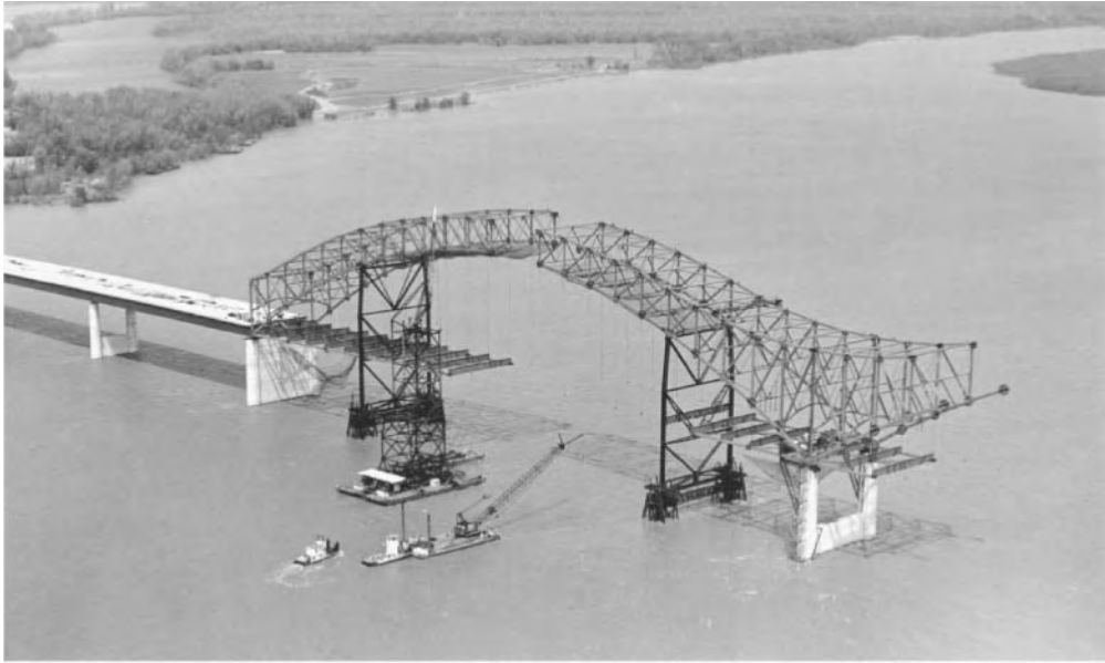
Figure 45.43 Erection of west arch span of twin-arch Hernando de Soto Bridge, Memphis, Tenn., 1972. The two 900 ft (274 m) continuous-truss tied-arch spans were erected by a high-tower derrick boat incorporating a pair of barges. West-arch steelwork (shown) was cantilevered to midspan over two pile-supported falsework bents. Projecting east-arch steelwork (at right) was then cantilevered to midspan (without falsework) and closed with falsework-supported other half-arch. (Courtesy of Bethlehem Steel Corporation.)
