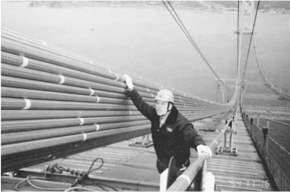
Figure 45.46 Parallel-wire strand main cable, Akashi Kaikyo suspension bridge, Kobe, Japan, 1994. The main span is 6532 ft (1991 m), by far the world's longest. The PWS at right is being towed across the spans, supported on rollers. The completed cable is made up of 290 PWS, making a total of 36,830 wires, and has a diameter of 44.2 in (1122 mm) following compaction — the largest bridge cables built to date. Each 127-wire PWS is about 2-3/8 in (60 mm) in diameter. (Courtesy of Nippon Steel — Kobe Steel.)
