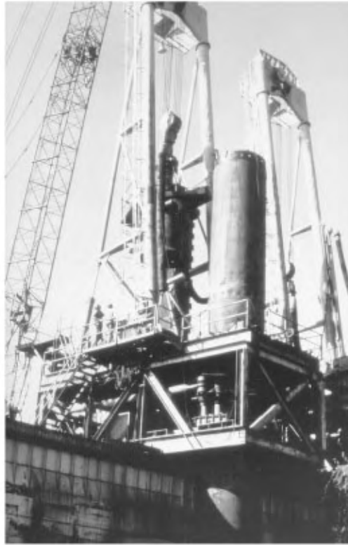
FIGURE 47.3 Steel tubular pile being installed from jack-up barge. Socket will be drilled into rock and entire pile filled with tremie concrete.
