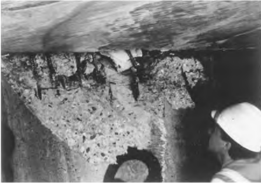
FIGURE 34.31 Damage to internal shear key in an abutment in the 1994 Northridge earthquake. (Source: EERI, Earthquake Spectra , Special Suppl. to Vol. II, 1995.)
