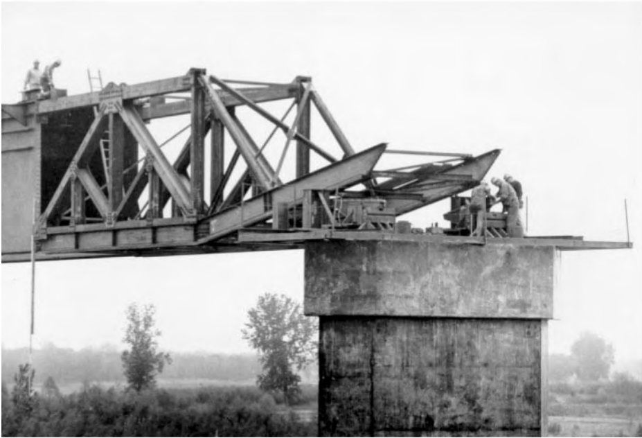
Figure 45.41b Launching nose rides up onto pier 5 skidway units, removing girder-train leading-end sag.
