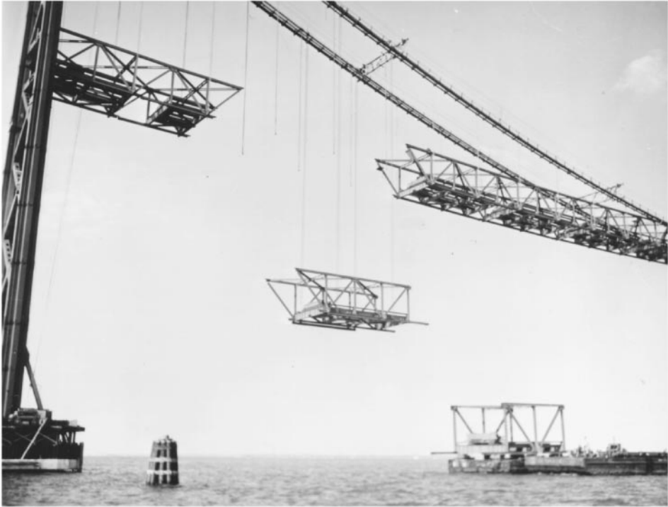
Figure 45.33 Erection of suspension bridge deck structure, first Chesapeake Bay Bridge, Maryland, 1952. A typical four-panel through-truss deck section, weighting 99 tons, has been picked from the barge and is being raised into position using four sets of lifting falls attached to main suspension cables. The closing deck section is on the barge, ready to go up next. (Courtesy of Bethlehem Steel Corporation.)
