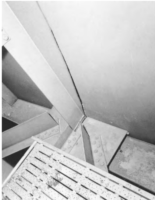
FIGURE 53.1 View of cracked girder of Lafayette Street Bridge in St. Paul, MN showing fatigue crack originating from backing bars and lack of fusion on the weld attaching the lateral bracing attachment plate to the web and to the transverse stiffener.
