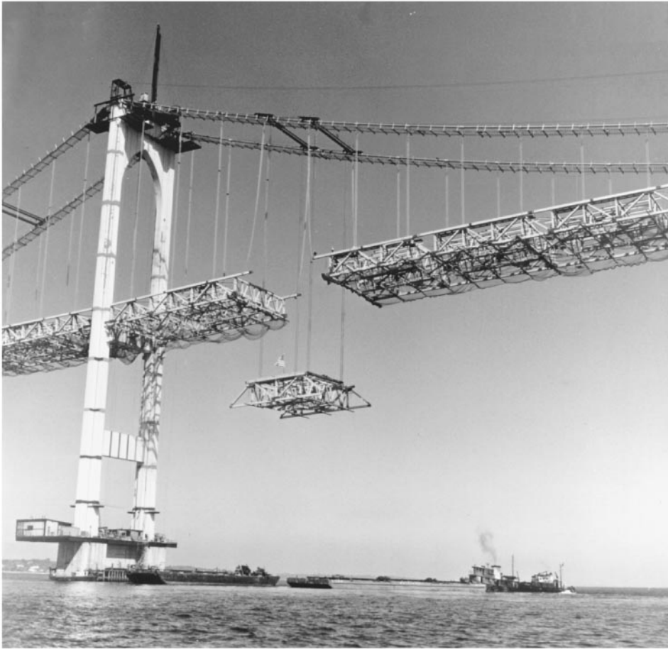
Figure 45.40 Suspended deck steelwork erection, the Newport Bridge suspension spans, Narragansett Bay, R.I., 1968. The closing mainspan deck section is being raised into position by two cable travelers, each made up of a pair of 36 in (0.91 m) wide-flange rolled beams that ride the cables on wooden wheels. The closing section is 40 1/2 ft (12 m) long at top-chord level, 66 ft (20 m) wide and 16 ft (5 m) deep, and weighs about 140 tons. (Courtesy of Bethlehem Steel Corporation.)
