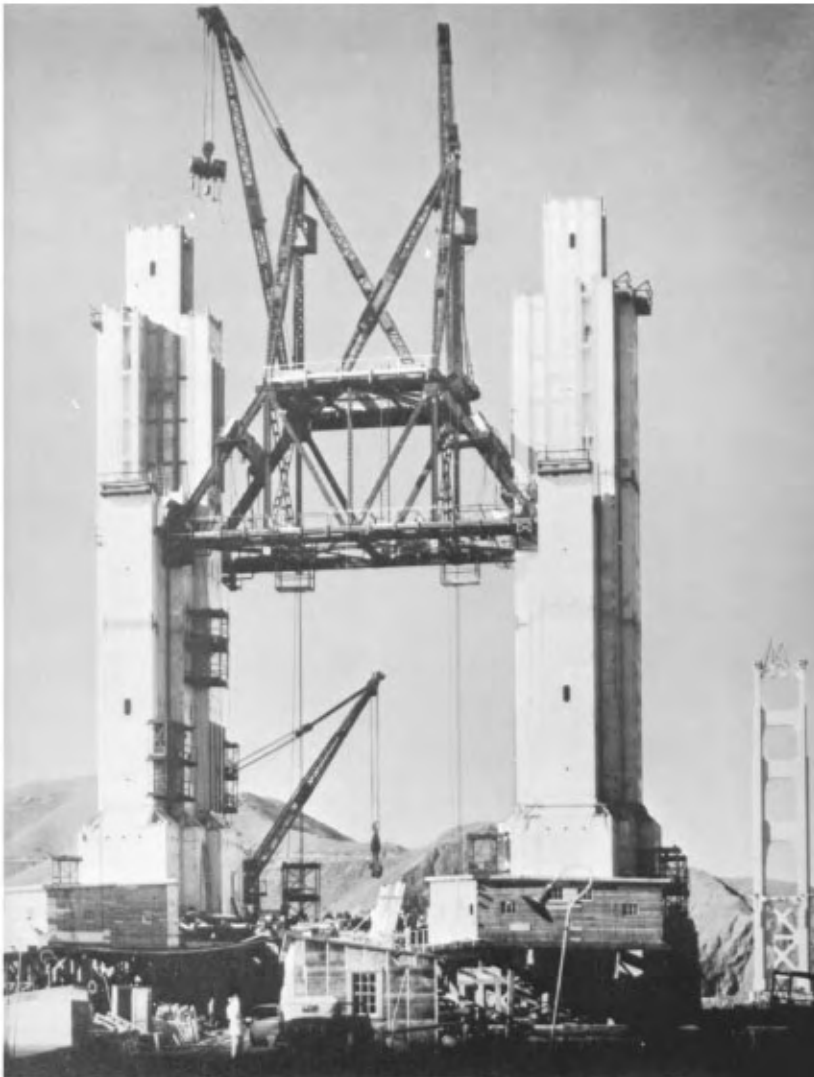
Figure 45.22 Erecting south tower of Golden Gate Bridge, San Francisco, 1935. A creeper traveler with two 90 ft (27 m) booms erects a tier of tower cells for each leg, then is jumped to the top of that tier and proceeds to erect the next tier. The tower legs are 90 ft (27 m) center-to-center and 690 ft (210 m) high. When the traveler completed the north tower (in background) it erected a Chicago boom on the west tower leg, which dismantled the creeper, erected tower-top bracing, and erected two small derricks (one shown) to service cable erection. Each tower contains 22,200 tons of steelwork.
