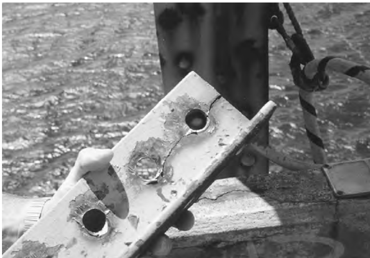
FIGURE 53.7 Connection angle from stringer to floor beam connection of a bridge over the St. Croix River on I-94 that cracked because it was too stiff.
