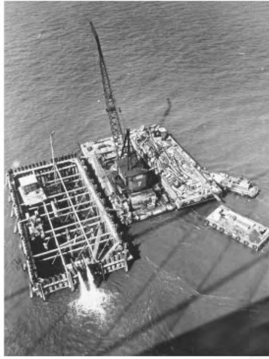
FIGURE 47.12 Dewatering the cofferdam for the main tower pier, Second Delaware Memorial Bridge.
