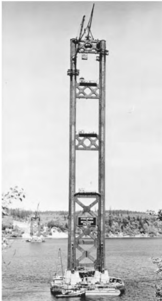
Figure 45.24 Tower erection, second Tacoma Narrows Bridge, Washington, 1949. This bridge replaced first Tacoma Narrows bridge, which blew down in a 40 mph (18 m/sec) wind in 1940. The tower legs are 60 ft (18 m) on centers and 462 ft (141 m) high. The creeper traveler is shown erecting the west tower, in background. On the east tower, the creeper erected a Chicago boom at the top of the south leg: this boom dismantled the creeper, then erected the tower-top bracing and a stiffleg derrick, which proceeded to dismantle the Chicago boom. The tower manhoist can be seen at the second-from-topmost landing platform. Riveting cages are approaching the top of the tower. Note tower-base erection kneebraces, required to ensure tower stability in free-standing condition (see Figure 45.27 ).
