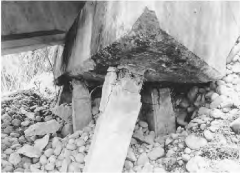
FIGURE 34.33 Abutment piles damaged during the 1991 Costa Rica earthquake. (Source: EERI, Earthquake Spectra , Special Suppl. to Vol. 7, 1991.)
