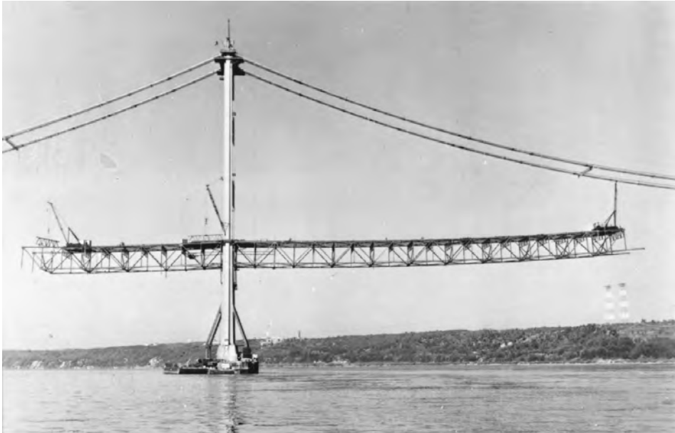
Figure 45.27 Erection of suspended deck steelwork, second Tacoma Narrows Bridge, Washington, 1950. The Chicago boom on the tower raises deck steelwork components to deck level, where they are transported to deck travelers by material cars. Each truss double panel is connected at top-chord level to previously erected trusses, and left open at bottom-chord level to permit temporary upward deck curvature, which results from the partial loading condition of the main suspension cables. The main span (at right) is 2800 ft (853 m), and side spans are 100 ft (335 m). The stiffening trusses are 33 ft (10 m) deep and 60 ft (18 m) on centers. Tower-base kneebraces (see Figure 45.24 ) show clearly here.
