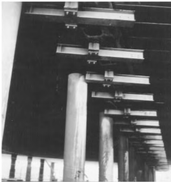
FIGURE 40.5 External hinge extenders on Santa Monica freeway structures.
