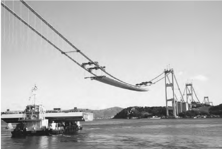
FIGURE 18.31 Block erection method on the Kurushima Kaikyo Bridge. (Courtesy of Honshu–Shikoku Bridge Authority.)
