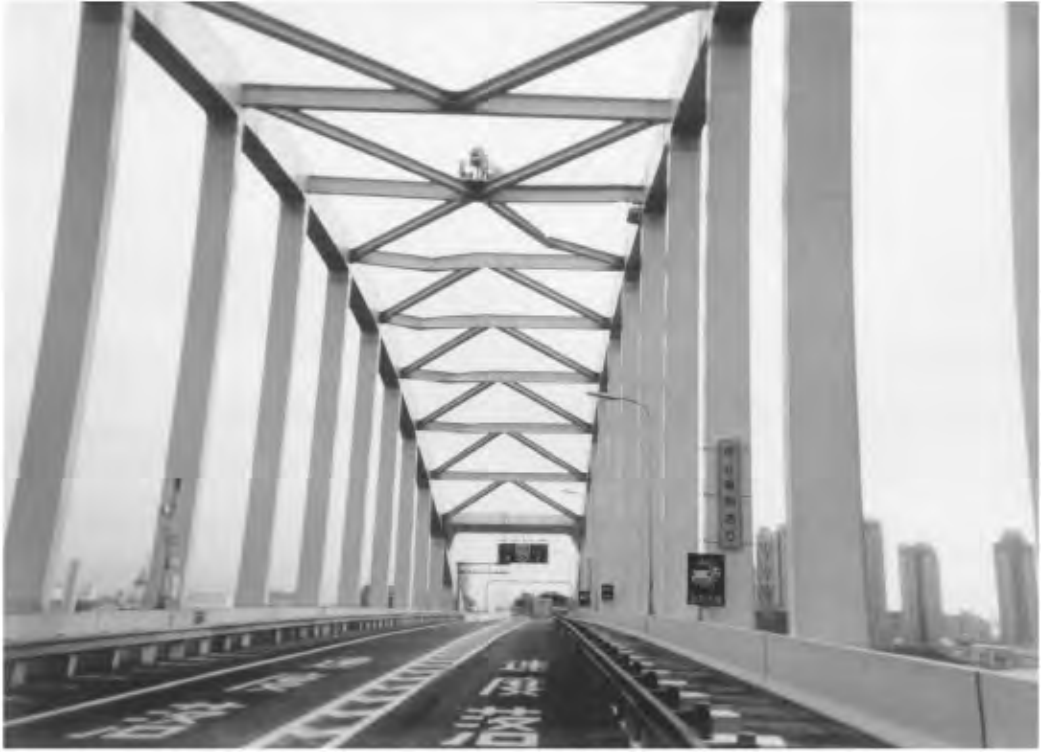
FIGURE 34.14 Buckling of cross-members in the upper chord of the Rokko Island Bridge in the 1995 Hyogo-Ken Nanbu earthquake.
