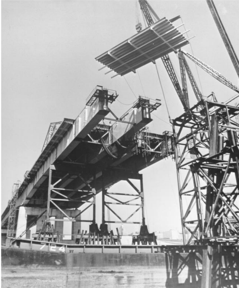
Figure 45.36 Erecting orthotropic-plate decking panel, Poplar Street Bridge, St. Louis, Mo., 1967. A five-span, 2165 ft (660 m) continuous box-girder bridge, main span 600 ft (183 m). Projecting box ribs are 5\frac{1}{2} \times 17 ft ( 1.7 \times 5.2 m) in cross-section, and decking section is 27 \times 50 ft ( 8.2 \times 15.2 m). Decking sections were field welded, while all other connections were field bolted. Box girders are cantilevered to falsework bents using overhead “positioning travelers” (triangular structure just visible above deck at left) for intermediate support. (Courtesy of Bethlehem Steel Corporation.)
