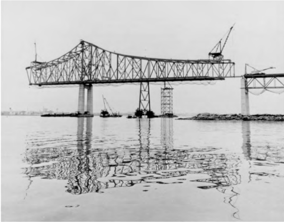
Figure 45.44 Closure of east side span, Commodore John Barry cantilever truss bridge, Chester, Pa., 1973. A high-tower derrick boat (in background) started erection of trusses at both main piers, supported on falsework; then erected top-chord travelers for main and side spans. The sidespan traveler carried steelwork erection to closure, as shown, and the falsework bent was then removed. The east-mainspan traveler then cantilevered the steelwork (without falsework) to midspan, concurrently with cantilever erection by the west-half mainspan traveler, and the trusses were closed at midspan. Commodore Barry has a 1644 ft (501 m) main span, the longest cantilever span in the U.S., and 822 ft (251 m) side spans. (Courtesy of Bethlehem Steel Corporation.)
