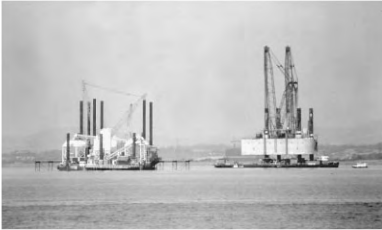
FIGURE 47.28 Installing precast concrete box caissons for Second Severn Crossing, Bristol, England. Extreme tidal range of 10 m and high tidal current imposed severe demands on installation procedures and equipment.
