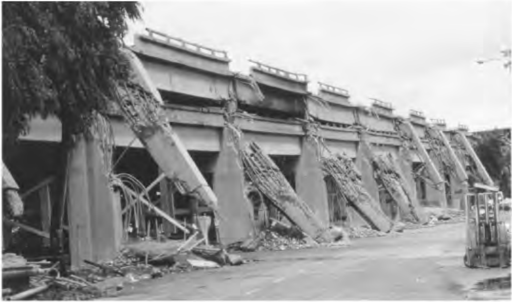
FIGURE 34.29 Cypress Street Viaduct collapse in the 1989 Loma Prieta earthquake.
