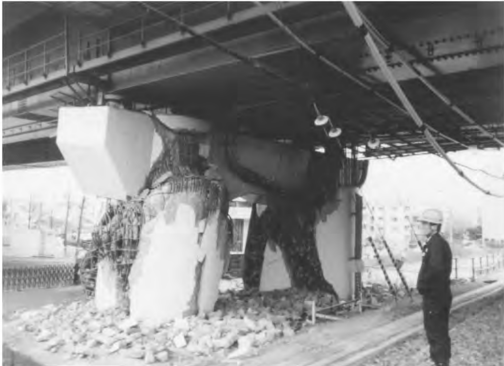
FIGURE 34.23 Failure of a two-column bent in the 1995 Hyogo-Ken Nanbu earthquake.
