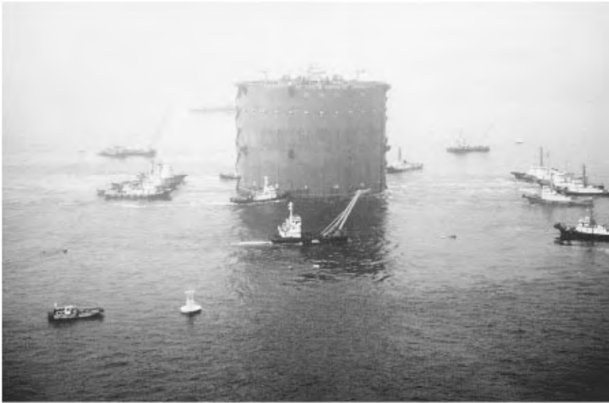
FIGURE 47.19 Steel box caisson being positioned for Akashi Strait Bridge, Japan, despite strong currents.
