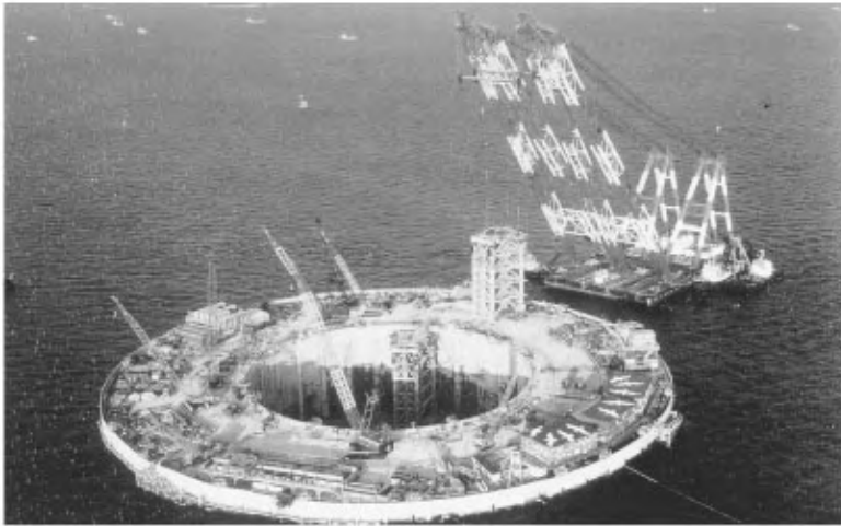
FIGURE 47.10 Slurry wall cofferdam for Kawasaki Island ventilation shaft, Trans-Tokyo Bay Tunnels and Bridge.
