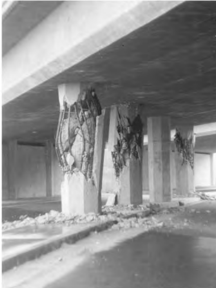
FIGURE 34.20 Failure of columns of the Route 5/210 interchange during the 1971 San Fernando earthquake.
