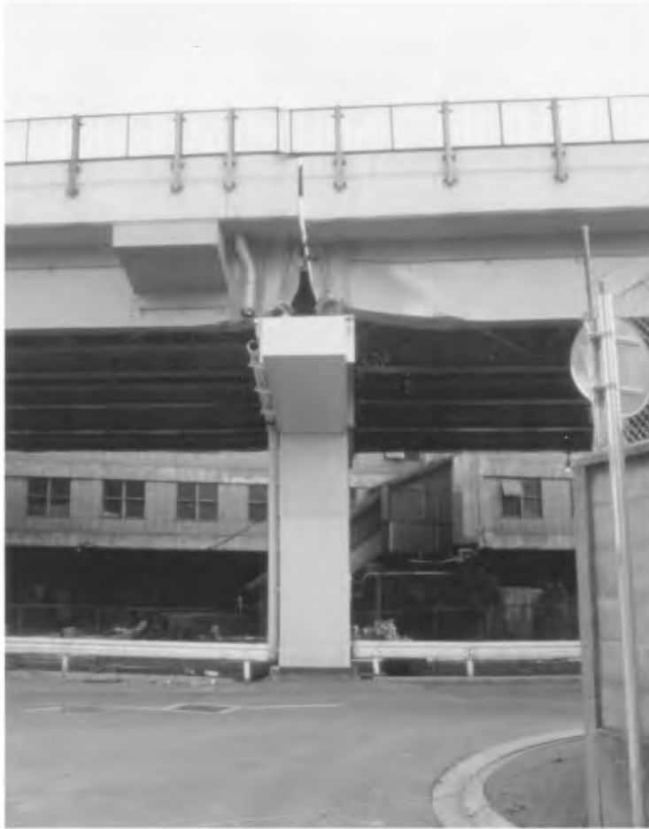
FIGURE 34.13 Girder damage at Bent 351 of the Hanshin Expressway apparently due to transverse movement during the 1995 Hyogo-Ken Nanbu earthquake.
