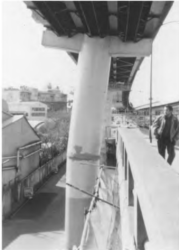
FIGURE 34.25 Local buckling of a circular cross-section column of the Hanshin Expressway in the 1995 Hyogo-Ken Nanbu earthquake.
