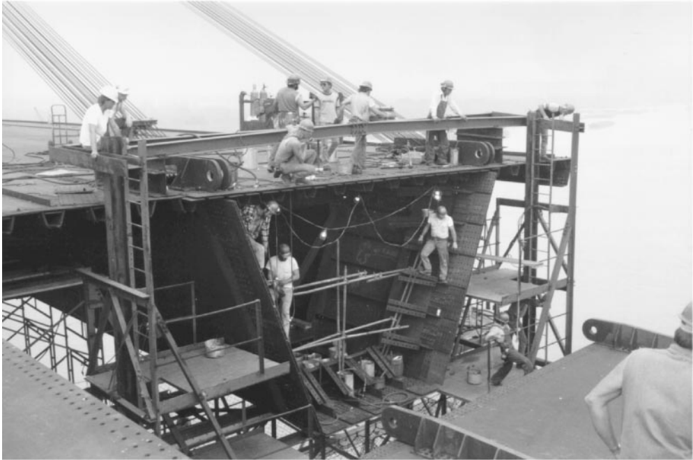
Figure 45.10 Luling Bridge deck steelwork erection, 1982; view looking northeast (refer to Figure 45.9 ). The twin box girders are 14 ft (4.3 m) deep; the deck plate is 7/16 in. (11 mm) thick. Girder section 16-east is being raised into position (lower right) and will be secured by large-pin hinge bars prior to fairing-up of joint holes and permanent bolting. Temporary erection stays are jumped forward as girder erection progresses.
