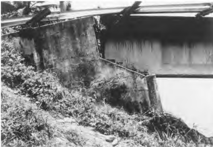
FIGURE 34.32 Rotation of abutment due to liquefaction and lateral spreading during the 1991 Costa Rica earthquake. (Source: EERI, Earthquake Spectra , Special Suppl. to Vol. 7, 1991.)
