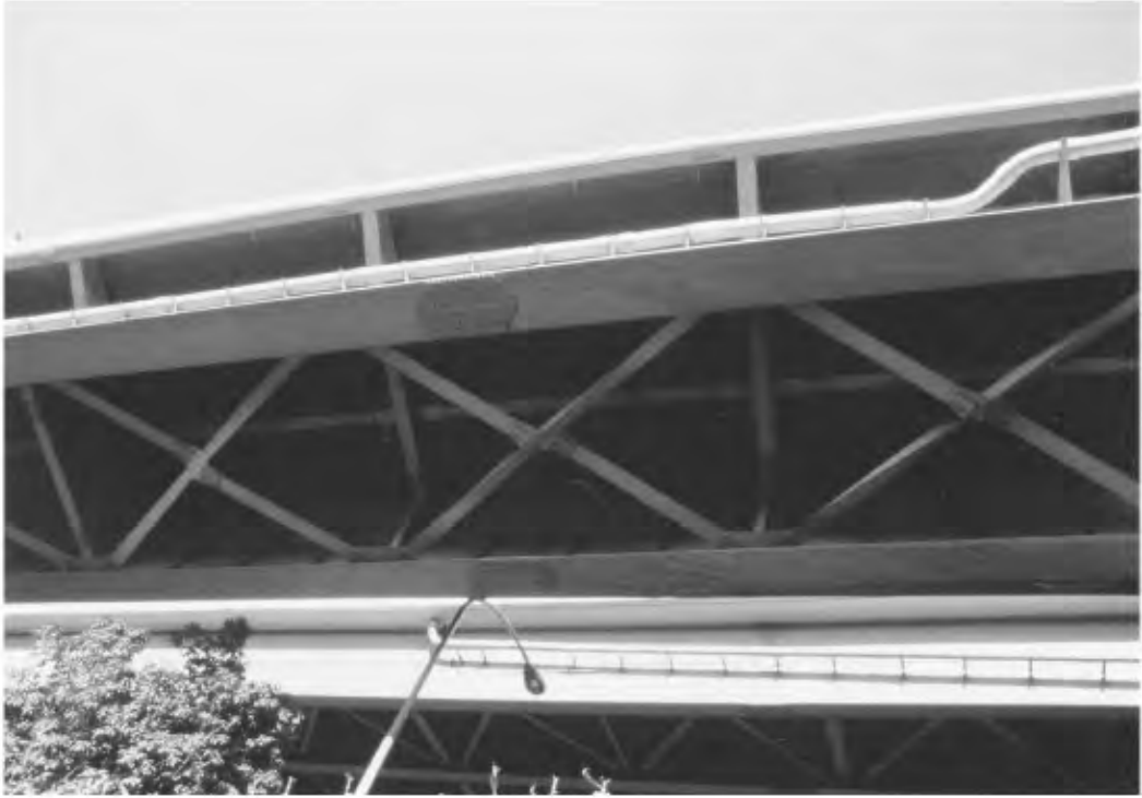
FIGURE 34.12 Buckling of braces near pier 209 of the Hanshin Expressway in the 1995 Hyogo-Ken Nanbu earthquake.
