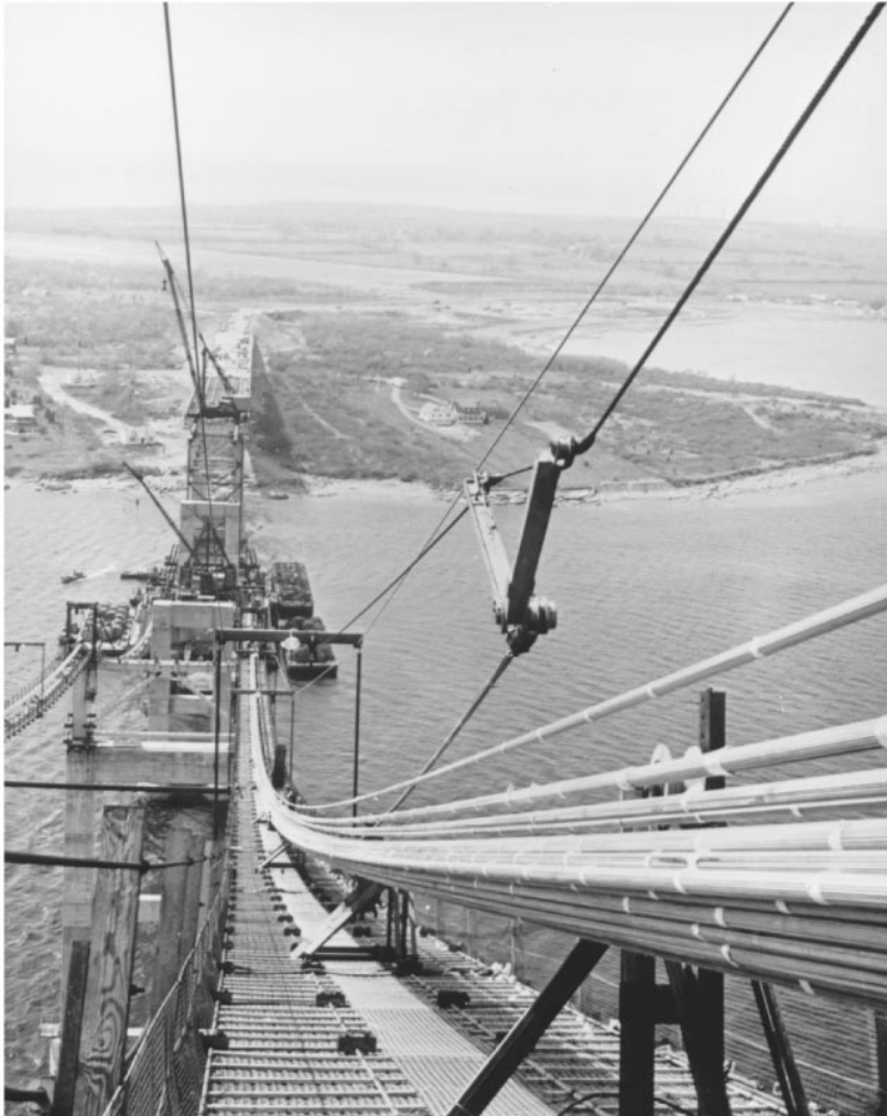
Figure 45.37a Aerial tramway tows PWS from west anchorage up side span, then on across other spans to east anchorage. Strands are about 1 3/4 in (44 mm) in diameter.
