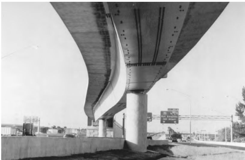
FIGURE 15.5 Single box girder bridge with integral bent cap — Ramp Y, I-95 Davies Blvd., Broward County, Florida.
