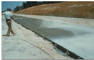
Spraying water or sealant - a chemical that forms a layer of membrane (film) that prevents evaporation
