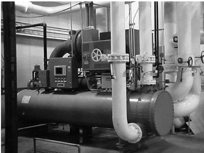
Figure 6-11. Picture of a Heat Recovery Chiller (source: Alabama Power Company)
