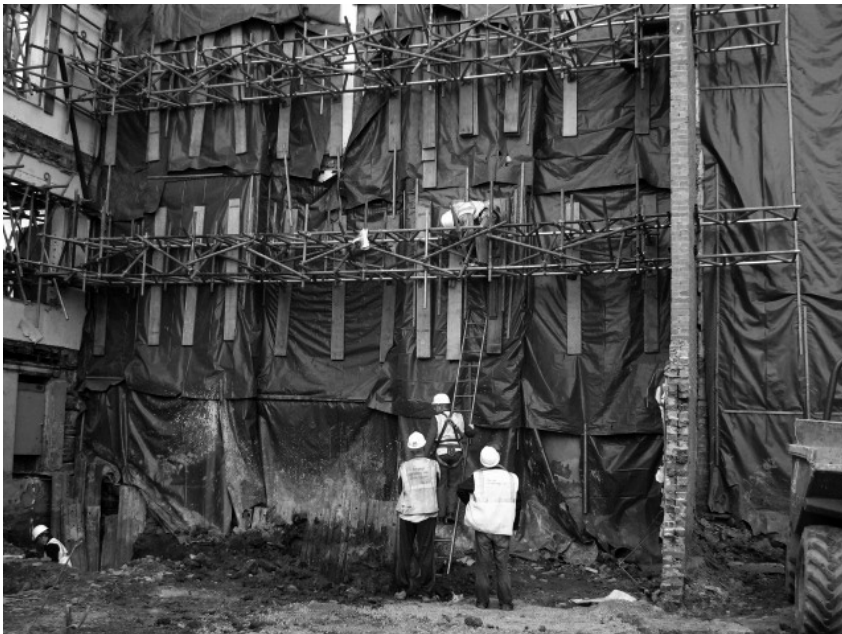
Photograph 12.6 Flying shores with scaffolding boards and plywood sheets provide support to a party wall; abutting wall constructed to provide lateral support
