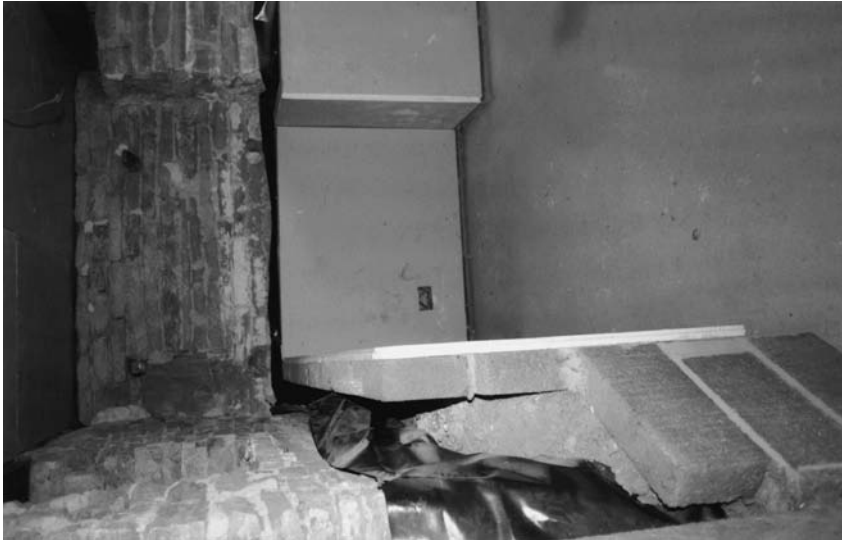
Photograph 6.3 Traditional dense polythene wall-lining with block-work loading wall and thermal-board dry lining. (Note: the untreated section of wall is above ground level)
