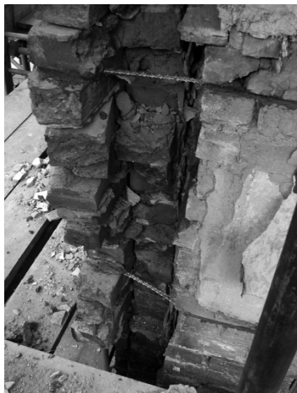
Photograph 12.2 Two-brick-thick solid wall reinforced with spiral cavity ties to prevent delamination of the brick wall
