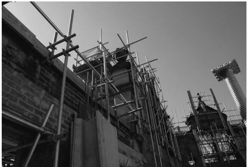
Photograph 13.30 East Brook Hall, Bradford: tubular scaffold system: clamps and through-ties secure ornamental features
