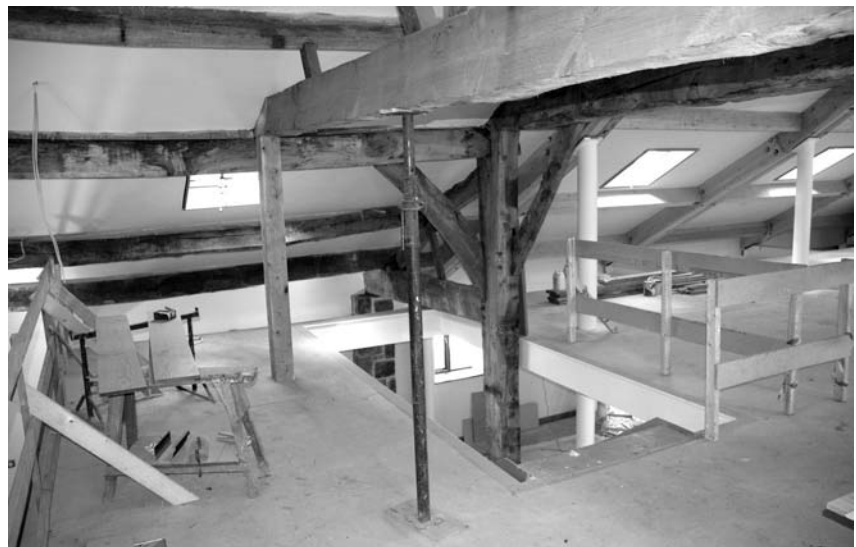
Photograph 7.4 Mezzanine floor introduced into a barn conversion making use of the large roof space
