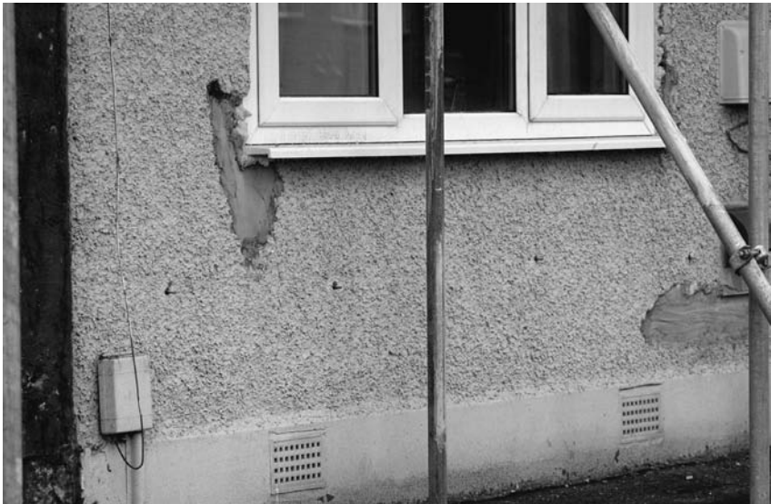
Photograph 12.1 Remedial cavity ties inserted: cracks in the render and structure have been filled and sealed with epoxy resin, ready to receive insulation and render
