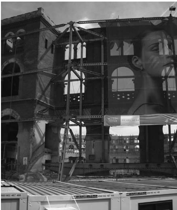
Photograph 13.9 Proprietary adjustable façade retention system
