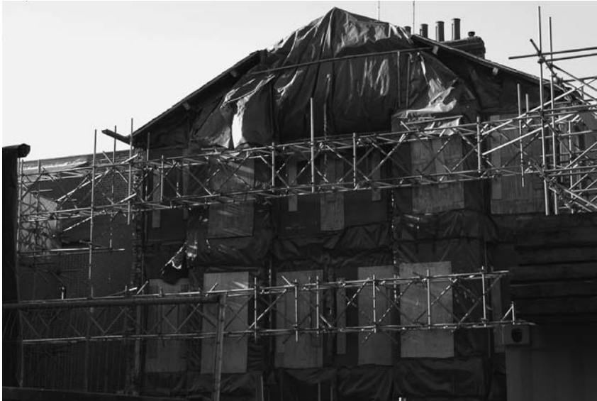
Photograph 12.5 Flying shores with scaffolding boards and plywood sheets provide support to a party wall
