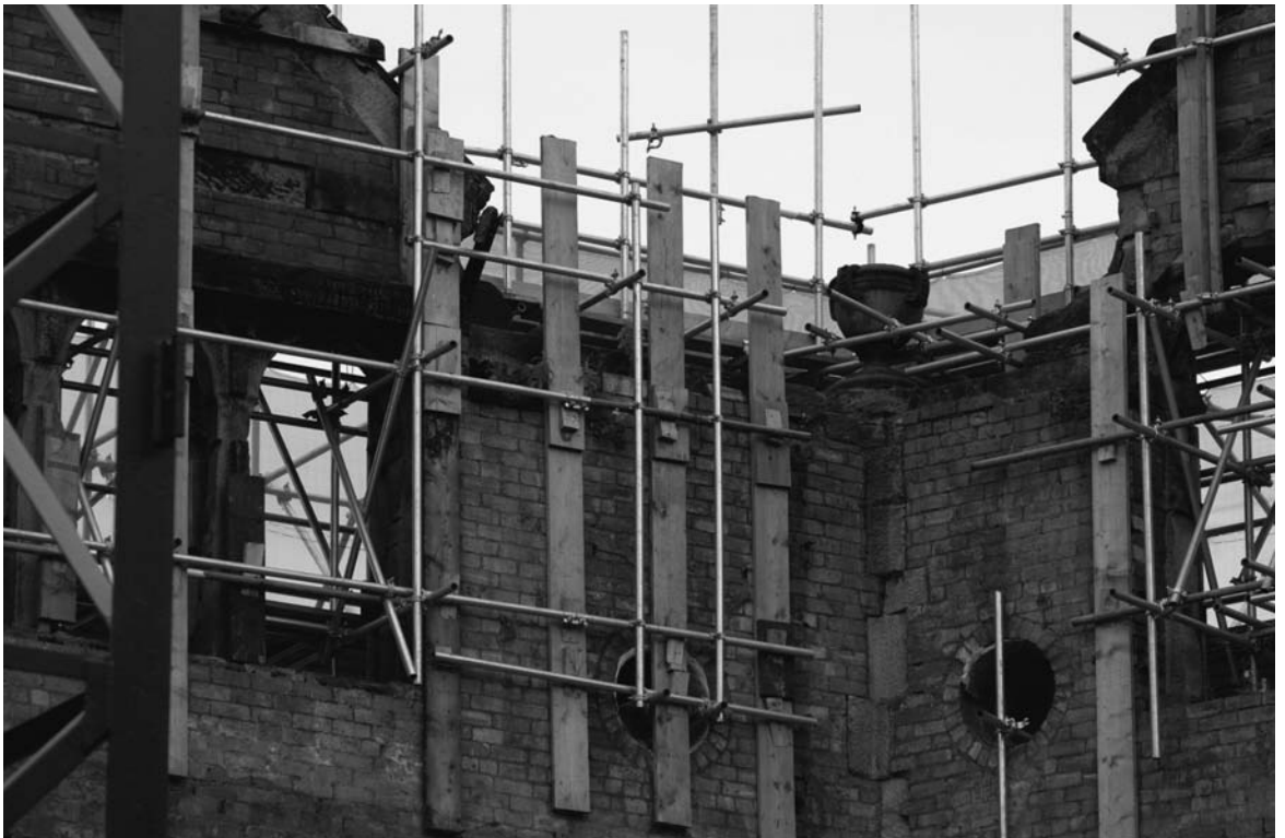
Photograph 13.32 East Brook Hall, Bradford: scaffolding boards are packed and wedged to ensure a firm fixing
