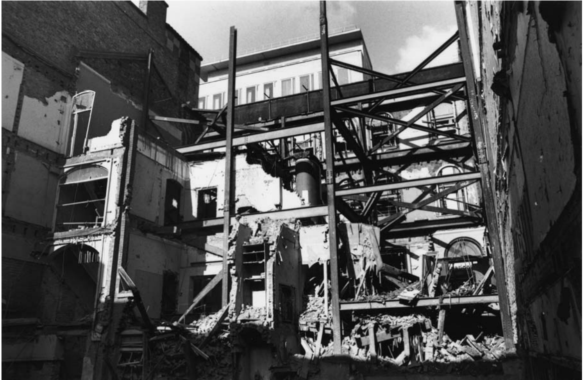
Photograph 13.13 Use of new steel frame to provide support; wholly internal façade support system
