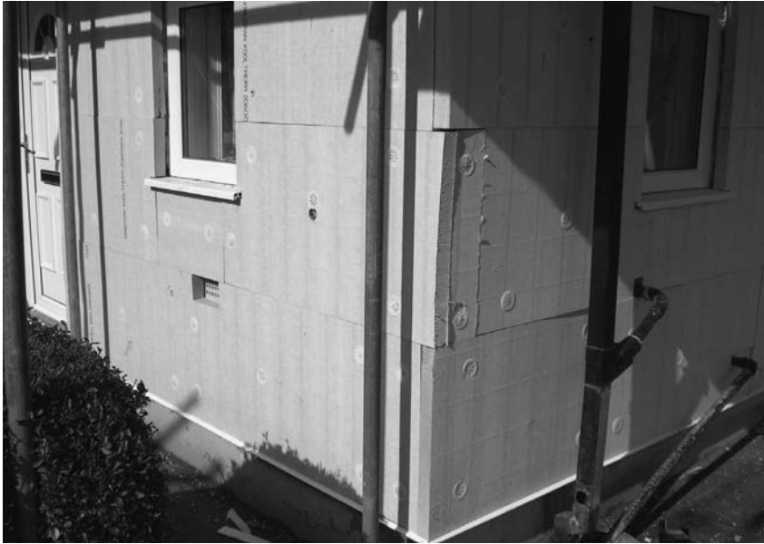
Photograph 4.3 Insulation trimmed around window openings and ventilation and cut to make corners
