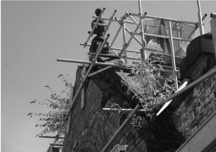
Photograph 13.31 East Brook Hall, Bradford: each ornamental feature may need to be individually supported and braced
