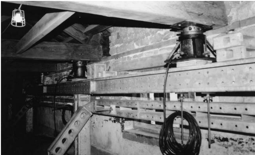
Photograph 10.2 The Granary Building, Leeds: temporary supports and jacks prior to lifting of roof
