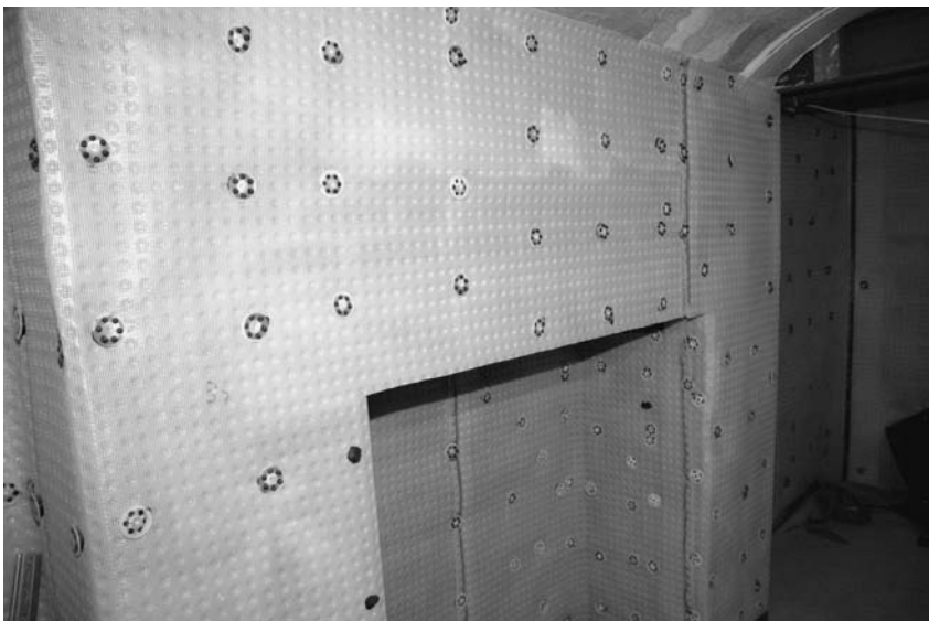
Photograph 6.2 Polypropylene cavity drain fixed with polypropylene studs ready to receive plaster finish
