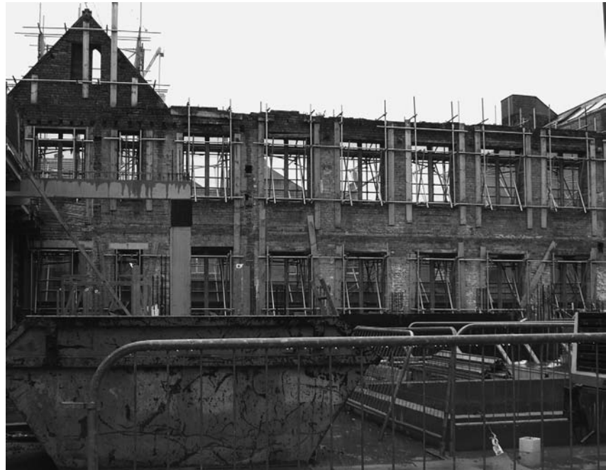
Photograph 13.6 Internal view of façade retention scheme at East Brook Hall, Bradford (cropped)
