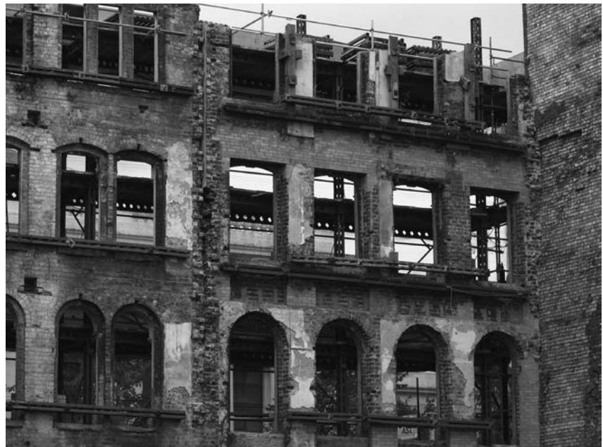
Photograph 13.23 Proprietary external façade support system, showing through-ties and straps across the internal face of the building, Belfast
