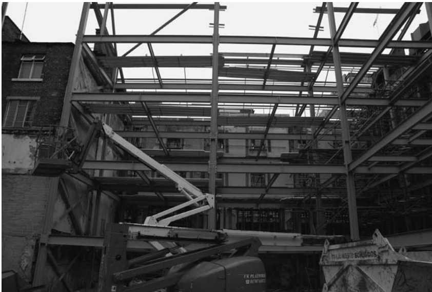
Photograph 13.2 Rear view of façade to row of terraces; shows new steel frame inserted behind façade
