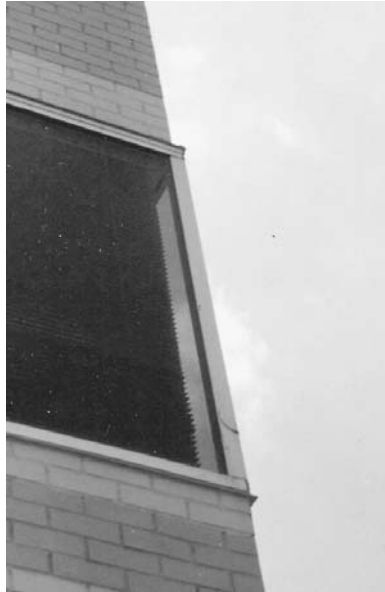
Figure 9-40 Protruding window invites leaks at head.
