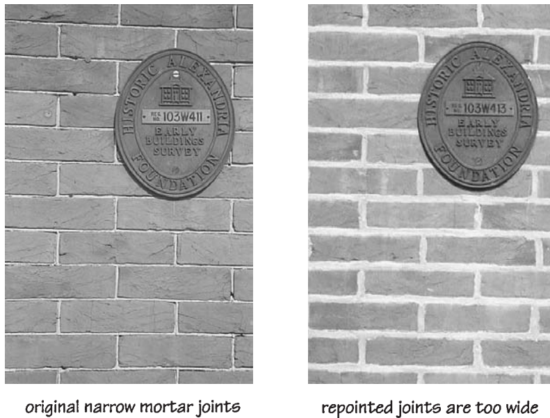
Figure 16-10 Original (left) and repointed (right) halves of building have very different appearance.
