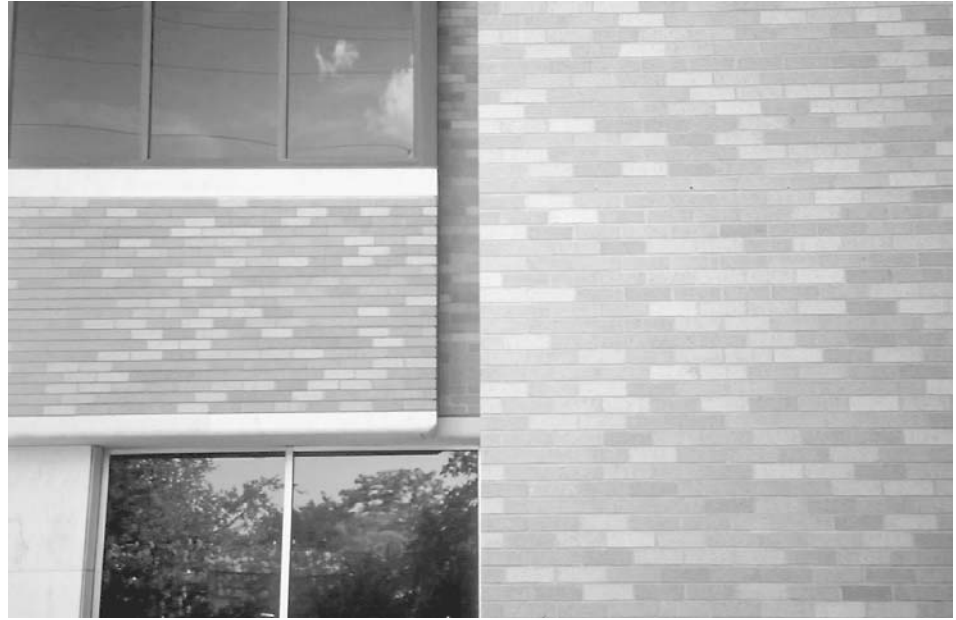
Figure 15-22 Raked horizontal joints in the wall panel on the left give the masonry a darker appearance than the concave tooled joints in the wall panel on the right.
