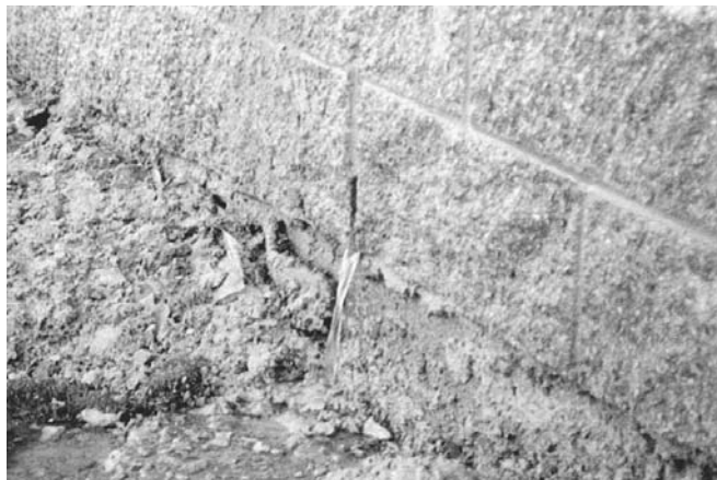
Figure 18-4 Water should drain immediately and freely from the weep hole immediately below the test location.
