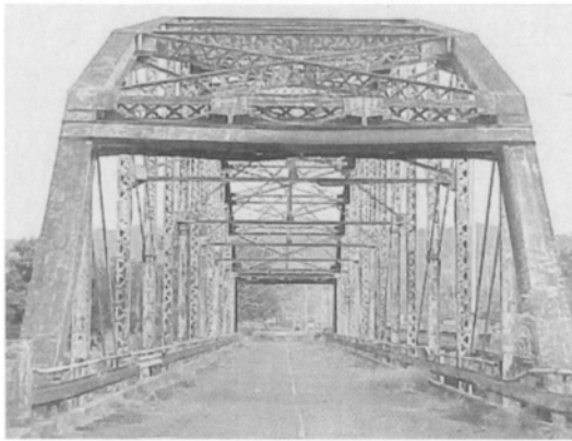
Figure 1.3 Uniform corrosion (atmospheric attack) of a steel bridge.
