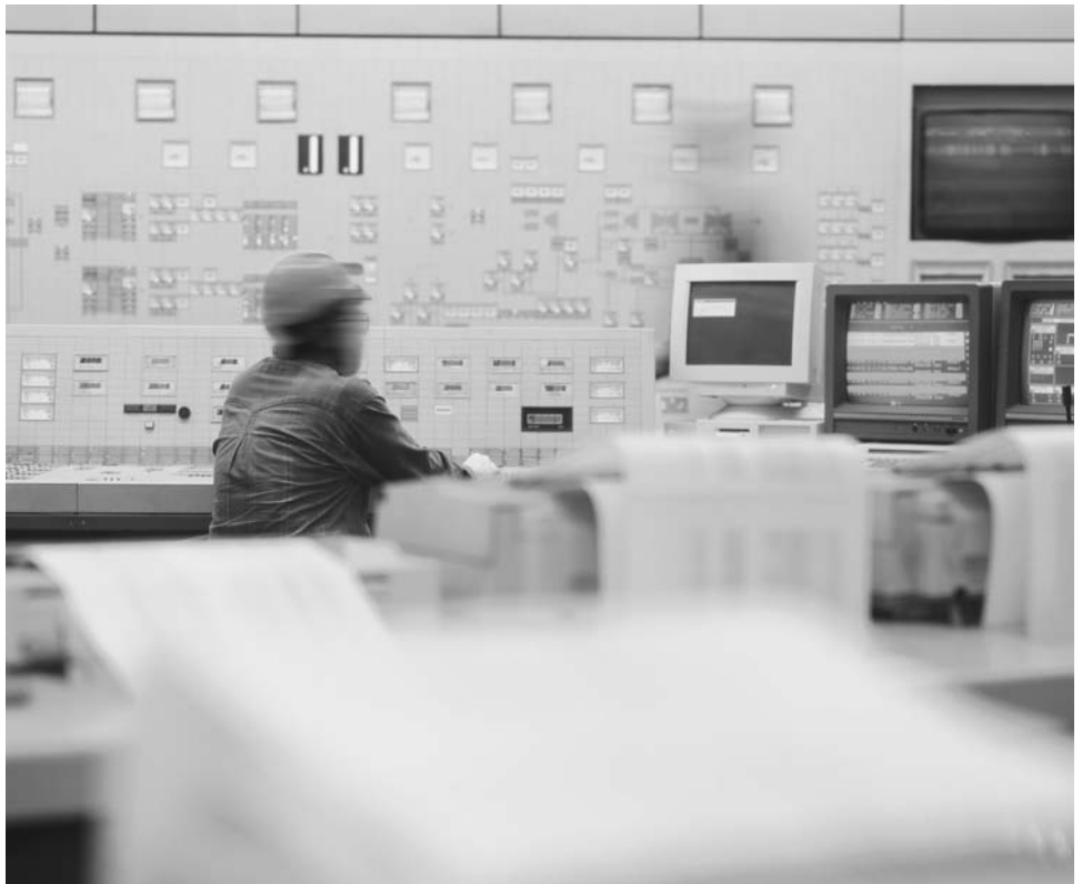
Figure 1.4 Typical industrial plant control room © Royalty-Free/Punchstock
