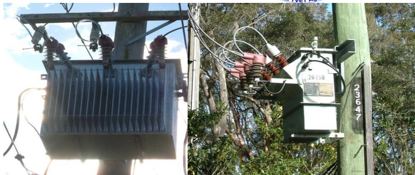
Fig. 10 TRANSFORMER TURN RATIO TEST
