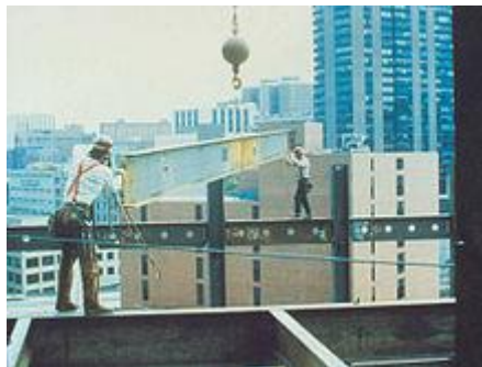
At-risk workers without appropriate safety equipment
