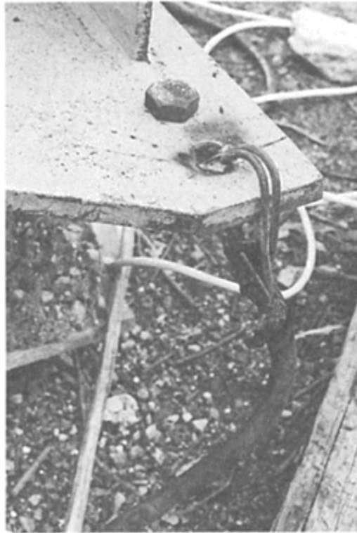
FIG. 10. A typical example of a poor and potentially hazardous site earth connection.
