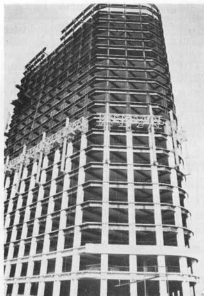
Figure 6.21 The America Tower, a 42-story composite building in Houston, Texas. Closely spaced exterior composite columns and moment-connected spandrel beams constitute a tube for resisting lateral loads. Note climbing form work on the exterior for composite exterior columns.
