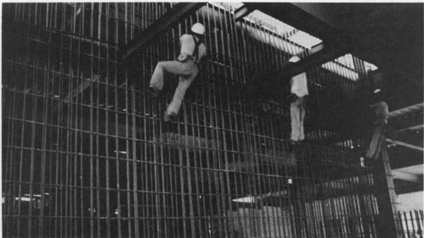
(c) Figure 6.1 Composite shear wall with steel beams. (a) Plan; (b) elevations; (c) photograph (note that steel beams run both parallel and perpendicular to shear wall).
