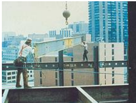
At-risk workers without appropriate safety equipment
