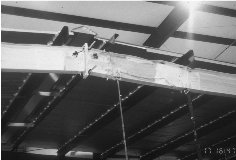
Fig. 8.41 Local buckling of flange. (Courtesy of Structures/Materials Laboratory, Virginia Tech.)
