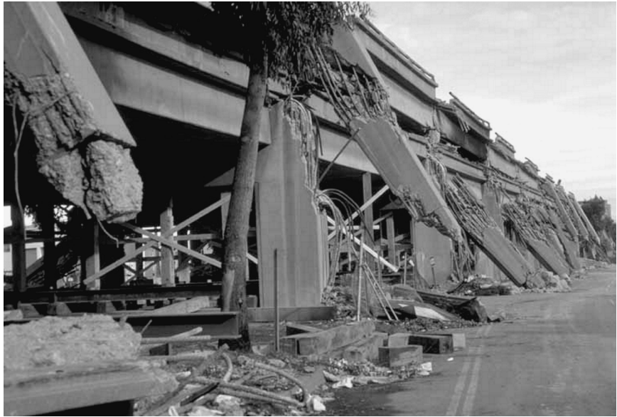
Fig. 1.26 Cypress Viaduct. (Photo courtesy H. G. Wilshire, U.S. Geological Survey.)
