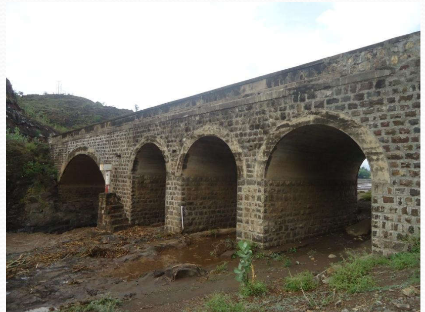
Jewha Bridge is constructed in 1938. The Bridge is located at 237.7Km from A.A in Robit- Ataye road segment.
