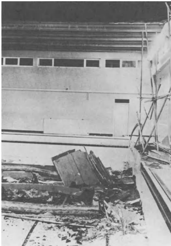
Fig. 2 The failure of a precast roof over a swimming pool at Stepney School, London
