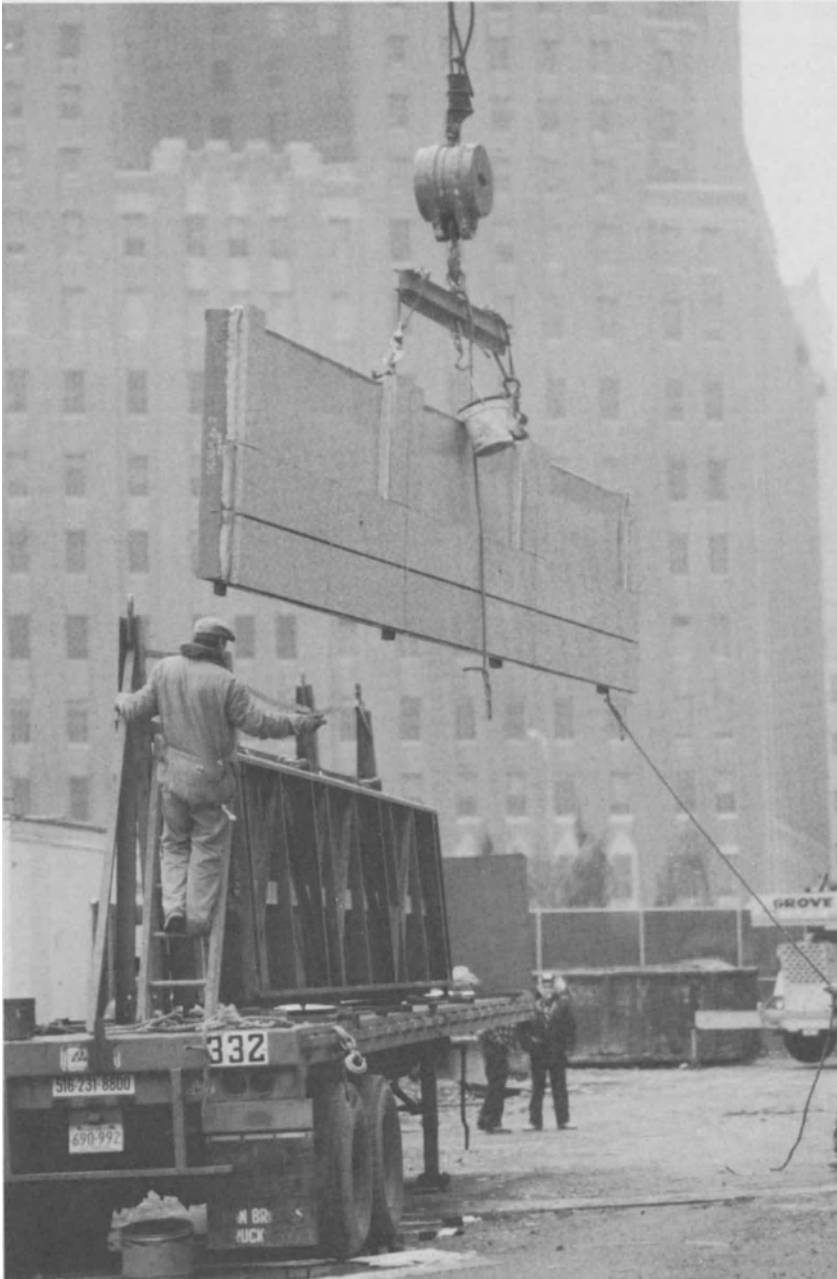
Fig. 3 Cranes were used to hoist materials in place directly from delivery trucks
