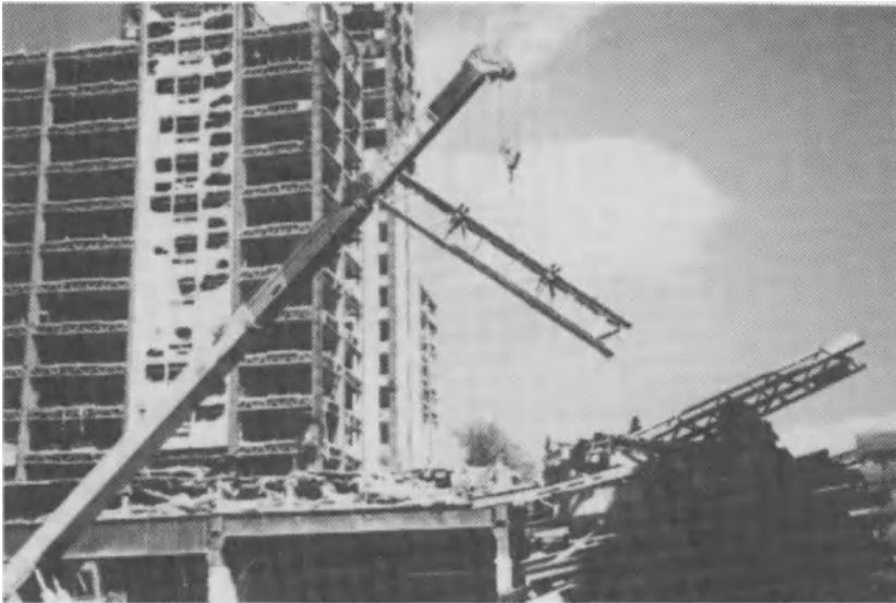
Fig. 4 Demolition of collapsed 21-story unit of Pino Suarez complex. 1985 Mexico City earthquake
