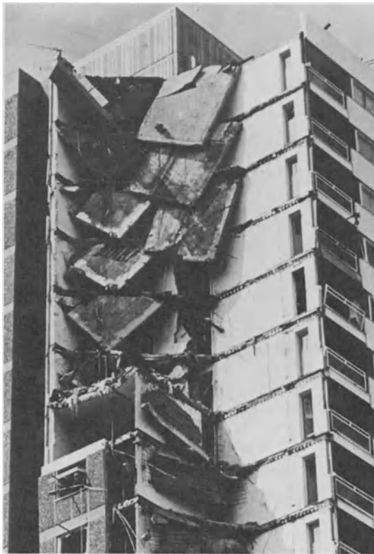
Fig. 1 The failure of a Large Panel System structure, Ronan Point, following a gas explosion 5 stories from the top of the building
