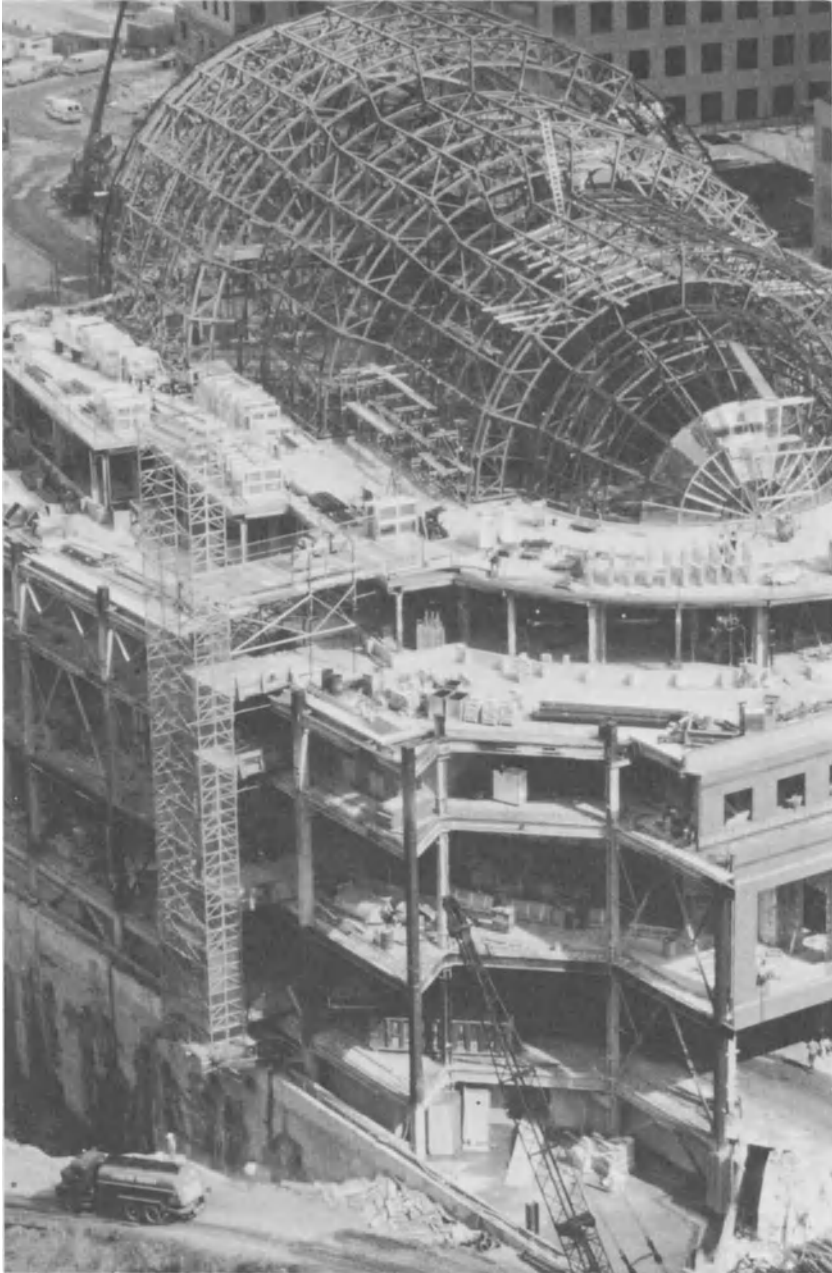
Fig. 9 Access roads, outside elevators, and cranes are all an important part of the construction process.
