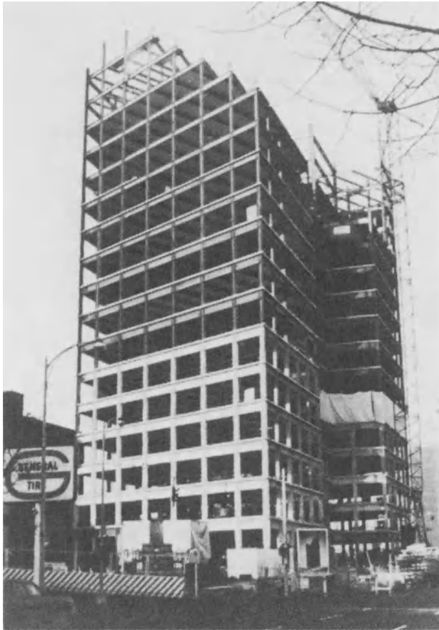
Fig. 10 Example of moment-resisting framing. Fourth and Blanchard Building, Seattle (Courtesy: United States Steel.)
