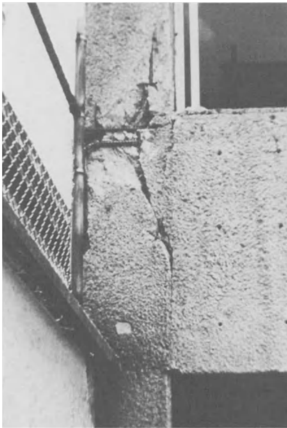
Fig. 4 Beam cracks in medical condominium building caused by the 1979 earthquake
