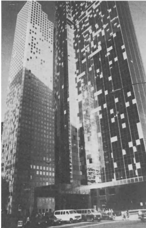
Fig. 2 Cladding damage to tall buildings in Houston, Texas (Hurricane Alicia, 1983)
