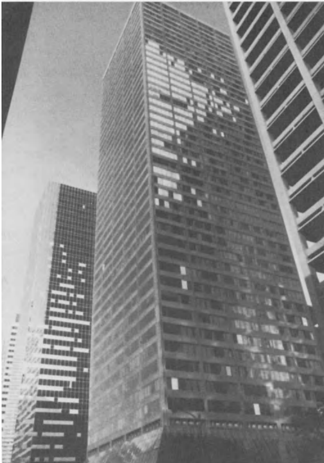
Fig. 1 Broken tempered glass fell from spandrels in Entex Building (background) while damaged annealed glass in vision areas remained in place (Hurricane Alicia, 1983)
