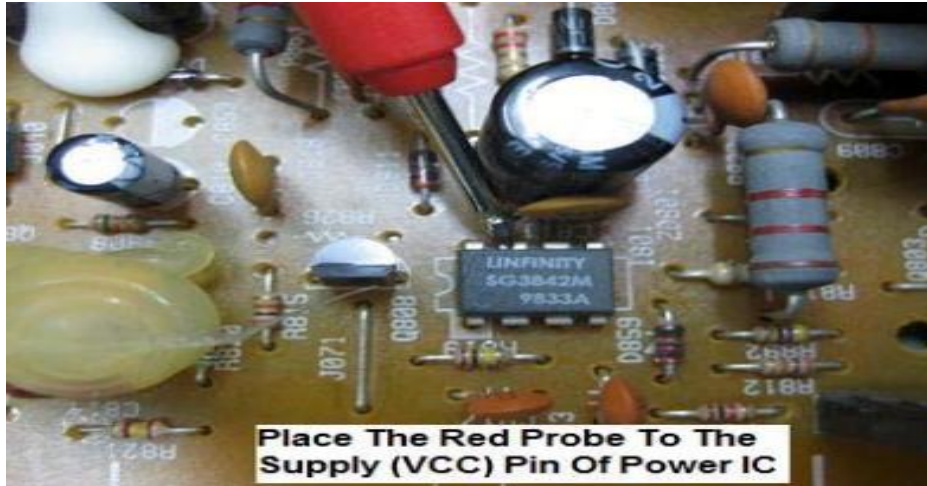
Figure3.20. Placing the RED test probe to the positive pin of the Filter Capacitor.
