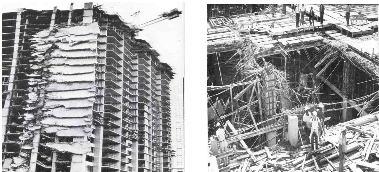
Fig. 5.10.8 Failure of formwork
