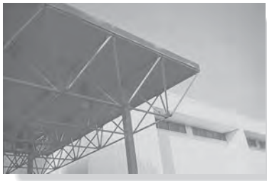
The roof of this pavilion is supported using a system of space trusses.
