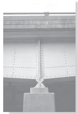
Typical pin used to support the steel girder of a railroad bridge.
