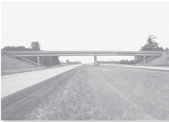
These bridge girders are statically indeterminate since they are continuous over their piers.
