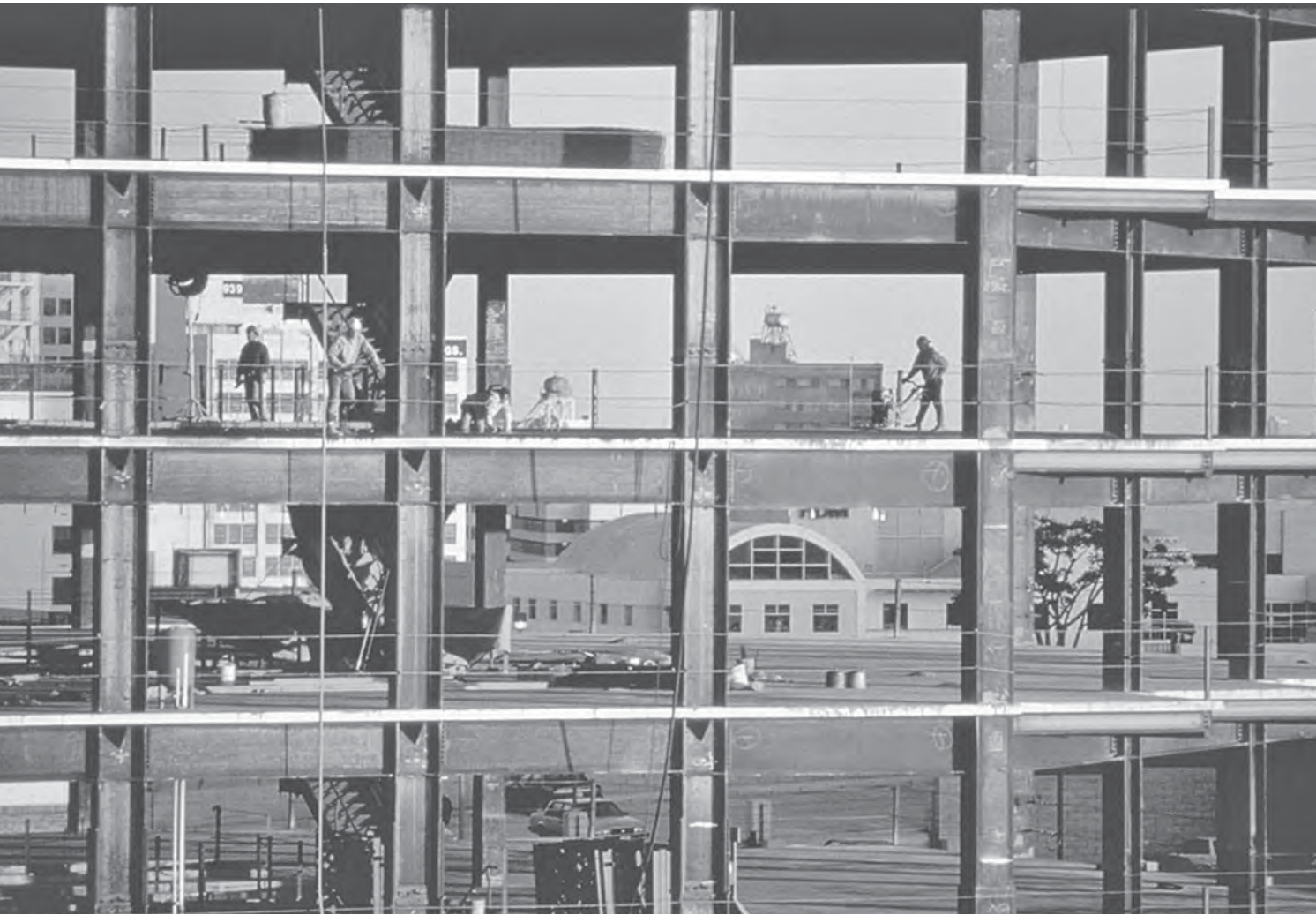
The fixed-connected joints of this concrete framework make this a statically indeterminate structure.
