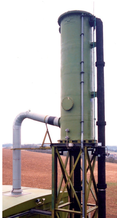
(c) Packed tower aerator of capacity 8 MI/day.
