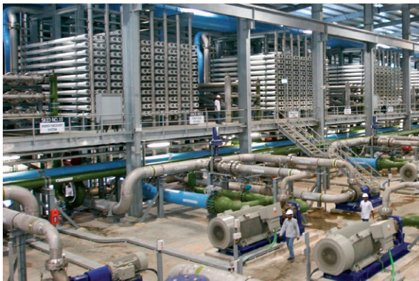
(b) Tuas SWRO plant (136 MI/d), Public Utilities Board, Singapore. (Black & Veatch consultant to EPC contractor, Hydrochem (S) Pte. Ltd.; developer: Hyflux Ltd.; operator: SingSpring Ltd.). (Photo: courtesy of Hyflux).
