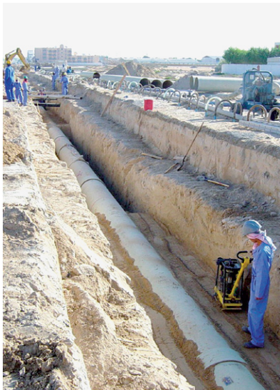
(c) 900 mm diameter GRP pipeline installation in Middle East—note attention to sidefill compaction. (Binnie Black & Veatch)
