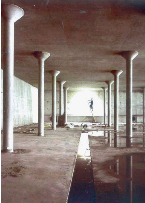
(a) Rectangular reinforced concrete monolithic service reservoir under construction in UK. (Engineer: Binnie & Partners)
