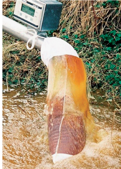
(b) Flushing a 100 mm diameter cast iron main. Debris collects in net for grading and analysis. Flow meter records the quantity of water used. (Black & Veatch)
