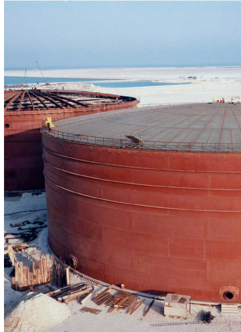
(b) 45 000 m 3 circular steel plate ground storage tanks under construction in the Middle East. (Engineer: Binnie & Partners).
