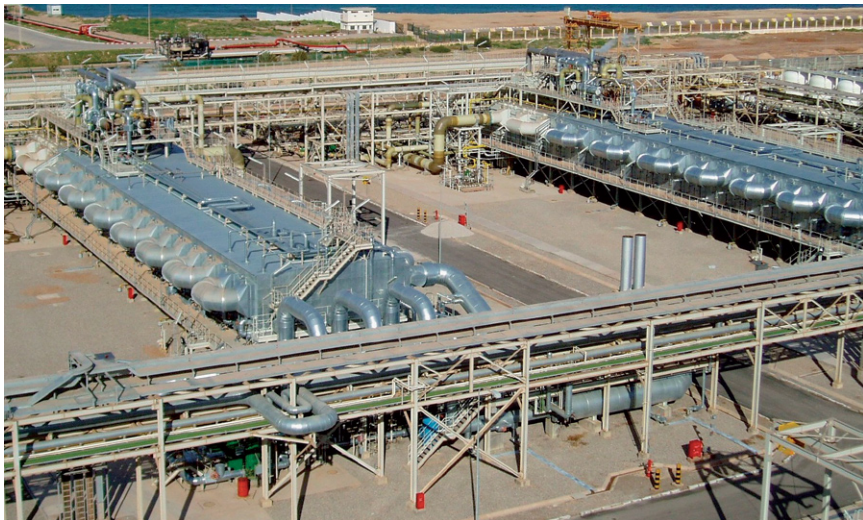
(b) 88 Ml/d multi-stage seawater flash distillation plant with 320 MW output on the Mediterranean coast. (Black & Veatch).
