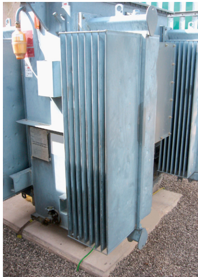
(a) Oil insulated transformer with gravel filled sump.
