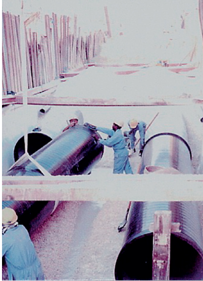
(a) Twin 1000 mm diameter ductile iron pipe laying in Middle East. (Black & Veatch)
