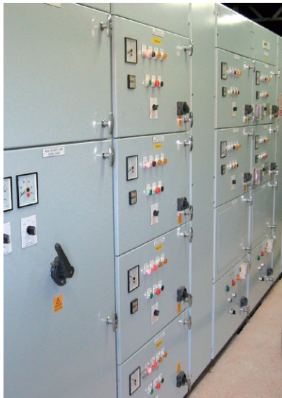
(b) MCC—sections from left to right: incomer and spare; 4 × plant motor starters; cable way; 2 × pump starters; 2 × pump starters.
