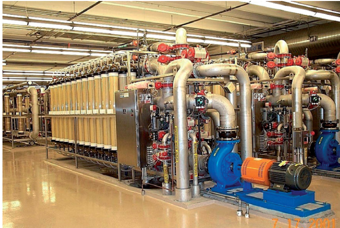
(b) Ultrafiltration membrane system for treatment of lime softened water, capacity 90 000 m 3 /day (Plant location: Mid West USA, System manufacturer: Koch Membrane Systems Inc., Wilmington, MA, USA).
