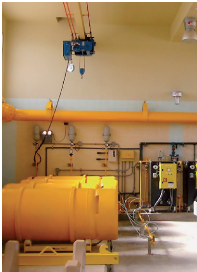
(a) Chlorine drum store with evaporator in the background. (Manufacturer: Portacel, UK; supplier: Bisan Inc. Canada.)
