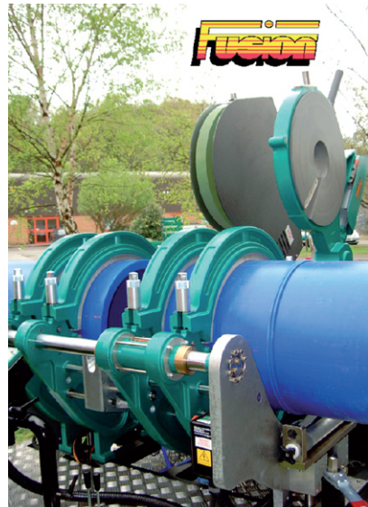
(d) Automatic butt fusion jointing of PE pipe. (Courtesy of The Fusion Group, Chesterfield, UK)
