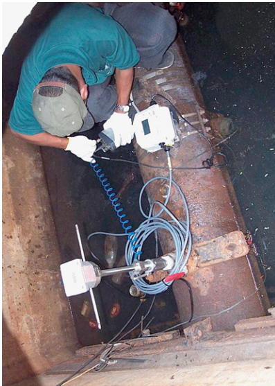
(c) Electromagnetic flowmeter insertion probe with pressure transducer and data logger. (Black & Veatch)
