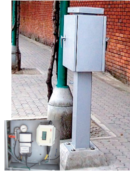
(b) District metering roadside cabinet. Control unit, data logger and pressure gauge. Telemetry and modem can also be installed. (Black & Veatch)
