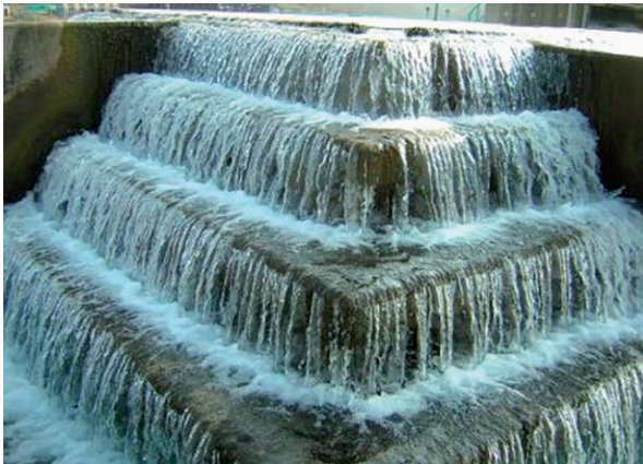
(b) A 4-step cascade aerator (each fall 0.5 m) for 2.75 m 3 /s flow rate at Izmit treatment works, Turkey. (Contractor: Paterson Candy Ltd. UK)
