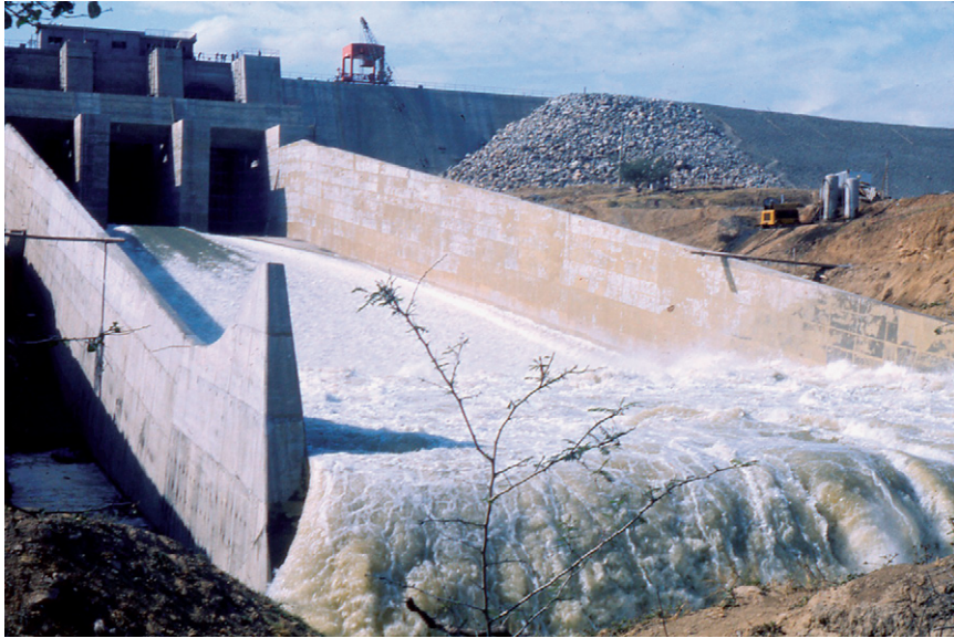
(a) Main spillway of 50 m high earth dam at Poechos, Peru—capacity 7200 m 3 /s.
