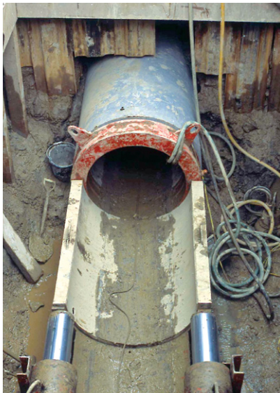
(c) Pipe jack under railway line for sleeve for 300 mm diameter trunk main. (Black & Veatch)
