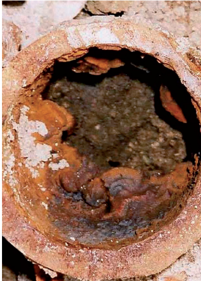
(a) Heavily tuberculated cast iron pipe. What is the value of pipe roughness?
