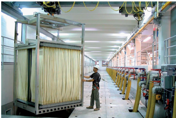
(b) Zenon ZeeWeed® 500d immersed membrane cassette being lowered into a tank. (Photo: GE Water and Process Technologies, Canada)
