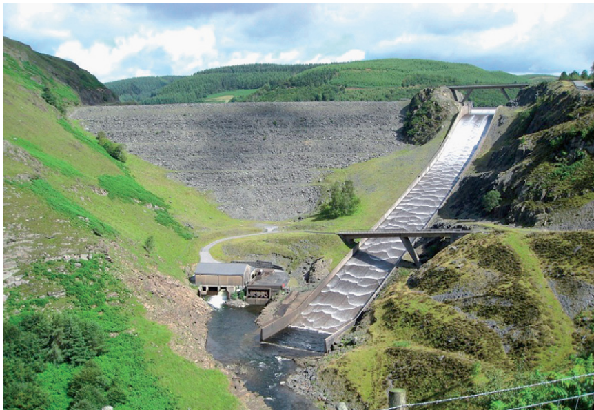
(b) Llyn Brianne 91 m high rockfill dam, Wales; side spillway: capacity 850 m 3 /s. (Courtesy of Aled Hughes) (Engineer: Binnie & Partners)
