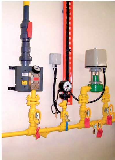
(b) Chlorine gas system with catchpot, changeover device and vacuum regulator. (Manufacturer: Portacel, UK)
