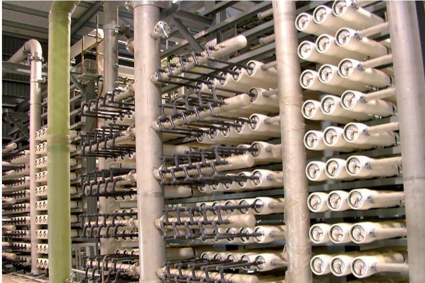
(a) Tuas SWRO plant, membrane units (see Plate 17(b) for credits).
