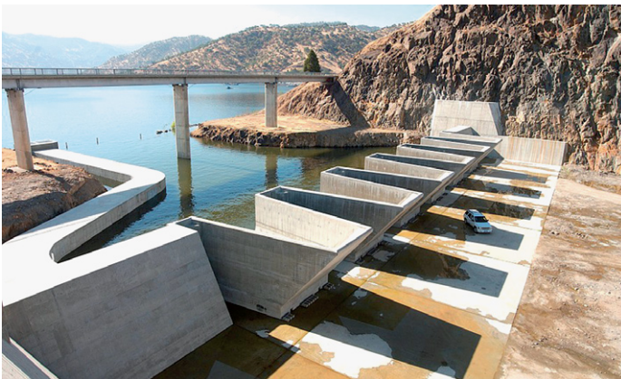
(c) Reinforced concrete labyrinth fusegates at Terminus Dam, California. Capacity 7545 m 3 /s after tipping of all gates. (Courtesy of Hydroplus, Inc, VA)
