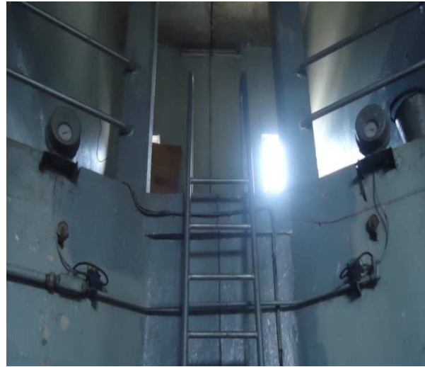
Figure 4.9 : Photo of Tank level measuring gauges
