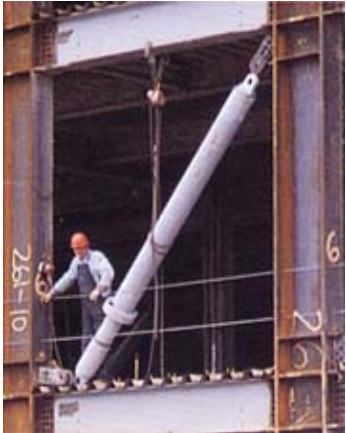
Viscous fluid damper installed in a building
