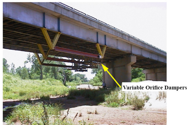
Variable orifice dampers installed on the I-35 Walnut Creek Bridge.
