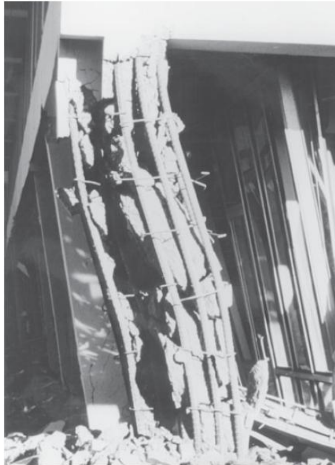
Fig. 11-6 Tied column destroyed in 1971 San Fernando earth- quake. (Photograph courtesy of National Bureau of Standards.)
