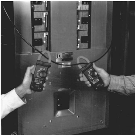
Figure 7.14 Average-responding rms to true rms ratio of less than 0.75. The meter on the left registers 59.2 and the meter on the right registers 40.5. (Reproduced with permission of Fluke Corp. ©.)
