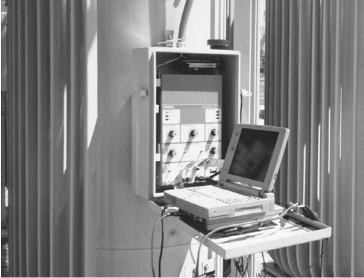
Figure 6.22 Flicker meter. (Courtesy of EPRI, PQTN Case No. 1, “Light Flicker Caused by Resistive Welder.”)
