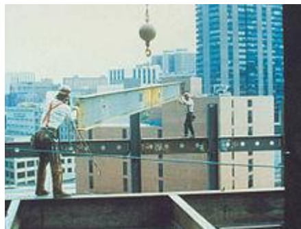
At-risk workers without appropriate safety equipment
