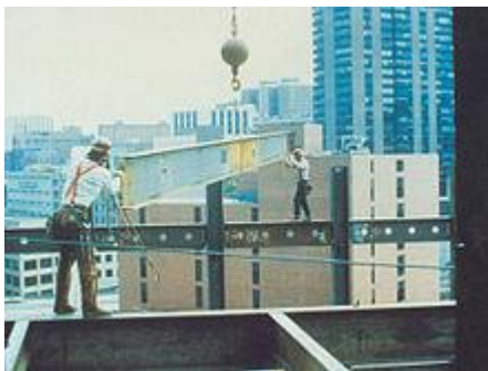
At-risk workers without appropriate safety equipment
