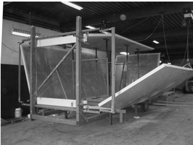
3.29 Assembly of sandwich panels into a monocoque Spacebox structure at Holland Composites Industrials.
