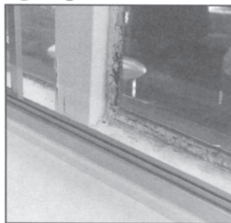
Are your windows old and rotten like these?
