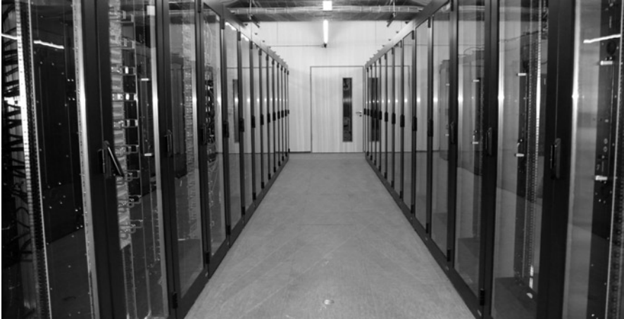
Fig. 6.62 A modern server room in a computing center of a university hospital
