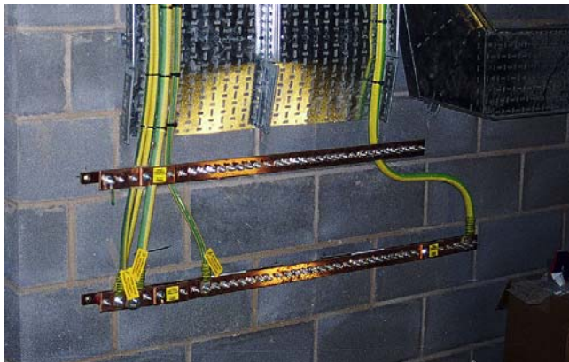
FIGURE 4.7 The main earth terminal in an industrial earthing location. The connections are located where inspection can readily be checked (W.T. Parker Ltd).
