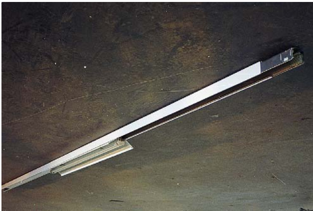
FIGURE 11.1 This type of lighting trunking has integral busbars carrying conductors for the supply to the luminaires. The 54-W twin fittings are available with either wide angle or semi-specular narrow beam characteristics, enabling effective lighting from different heights. The trunking can be suspended from the building frame and, with the narrow beam reflectors, is suitable for high-bay illumination. The clip-in fittings can be arranged to pick up from different phases and the whole assembly can be carried out without the use of tools, a particular advantage when working at heights (W.T. Parker Ltd).
