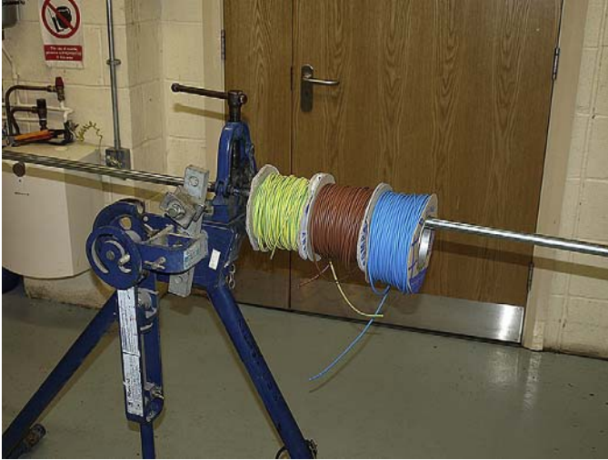
FIGURE 9.16 Running off cables from reels. Illustrates a typical method used when only a few cables are involved. A short piece of conduit is gripped in a pipe vice. When many reels have to be handled it is best to use a special rack.
