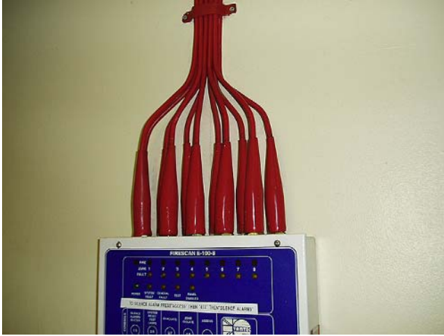
FIGURE 14.1 Control wiring in 3 \times 1.5\text{mm}^2 PVC-sheathed MI cable (Wrexham Mineral Cables).
