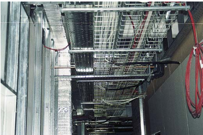
FIGURE 8.4 A high-level cable route in an industrial building is illustrated in this view. Cable ladder is provided to carry distribution cables feeding switchboards remote from the site sub-station. Cable basket, which in this case has three separate compartments, is to be used for data cabling and cable tray is provided for final circuits feeding lighting and machinery (W.T. Parker Ltd).
