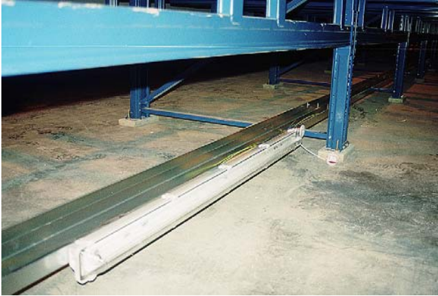
FIGURE 8.1 Emergency lighting fittings used in this warehouse stacking system are mounted at floor level on multi-compartment trunking. This enables separation of circuits of different voltage bands (W.T. Parker Ltd).
