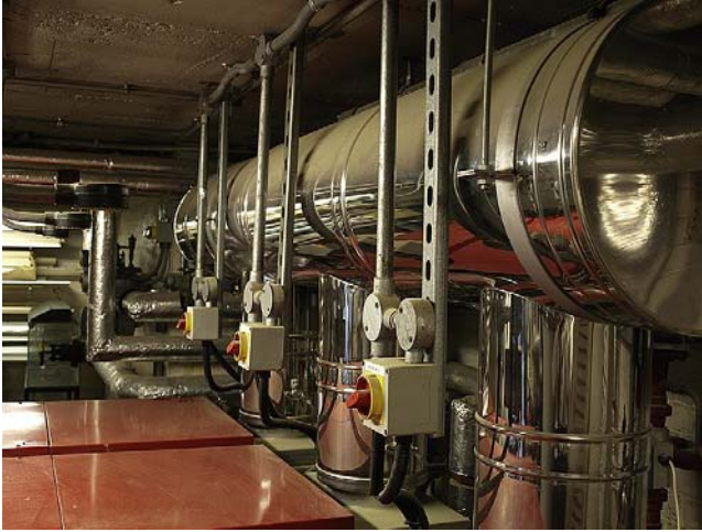
FIGURE 8.5 Wiring systems in use in a boiler house. The main wiring is in steel conduit and short lengths of heat-resisting cable in flexible conduit are used for the connections in the vicinity of the boiler where the temperatures are high (M.W. Cripwell Ltd).
