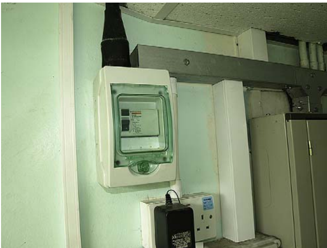
FIGURE 5.10 A 63-A RCCB with a 30-mA tripping current is fitted in a school and protects specific parts of the installation.
