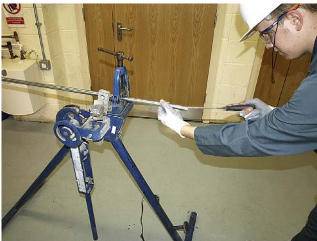
FIGURE 9.8 Conduit should be cut using a hacksaw and after cutting and threading any burrs should be removed using a file.
