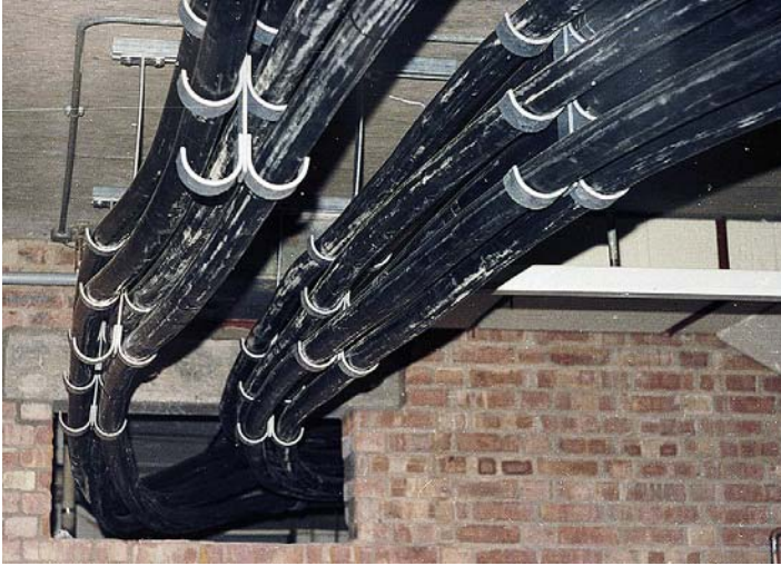
FIGURE 8.2 PVC/SLWA/PVC sheathed cables being used as sub-main cables for distribution of power. Provision has been made for 12 240mm 2 four-core cables to be run, and in this view 11 have been fitted (William Steward & Co Ltd).
