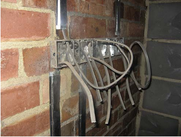
FIGURE 13.1 A kitchen ring main being installed in a dwelling house using concealed wiring. Steel capping has been secured in the permitted positions (Fig. 13.7) and the outlet boxes have been secured and cable installed prior to plastering taking place (NBK Electrical).
