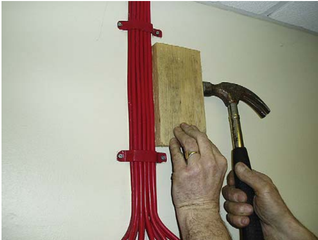
FIGURE 14.2 Straightening up multiple runs of MI cable using a block of wood and hammer (Wrexham Mineral Cables).
