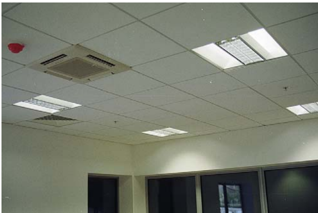
FIGURE 15.4 Suspended ceilings are regularly encountered in commercial premises. The matrix is designed to accept air conditioning, fire detection and lighting fittings, as seen in this view. The luminaires are Dextra compact fluorescent fittings with reflectors which give indirect as well as direct illumination (W.T. Parker Ltd).
