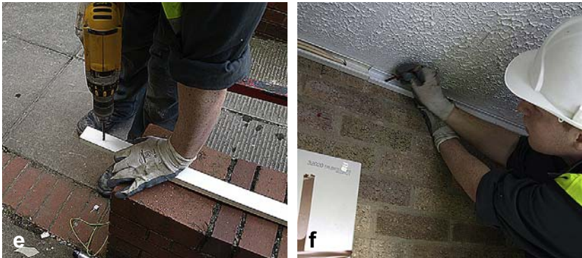
(e) Fixing holes are required and these are next drilled at suitable positions. (f) After drilling the conduit, the wall is correspondingly marked out and drilled for wall plugs.
