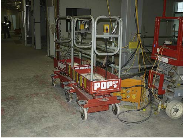
FIGURE 1.3 Battery powered re-chargeable working platforms in use in a new building greatly help in carrying out installation work at heights. The units are stable on level ground, have protection devices fitted and can easily be set by the operator to the most convenient working height (M.W. Cripwell Ltd).
