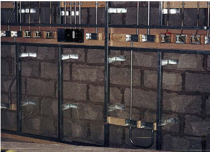
FIGURE 9.21 A neat completed conduit installation, ready for wiring to be installed (William Steward & Co. Ltd).
