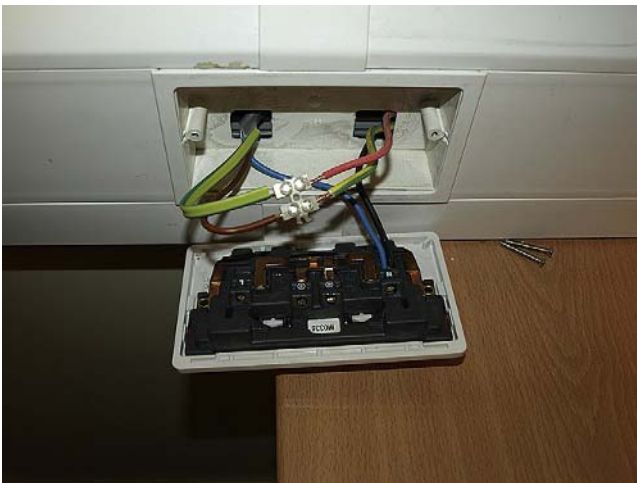
FIGURE 16.1 The test for continuity involves using a bridging strap connected between the line conductor and the relevant earth connection related to the particular circuit, here conveniently applied at a socket outlet.
