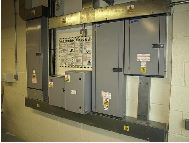
FIGURE 5.8 A distribution board in use in a college premises. The board incorporates three MCB distribution panels and associated switches. The installation is neatly wired in steel trunking and on cable tray.
