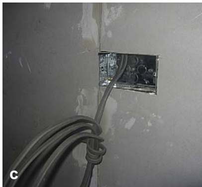
(c) After the wall surface is complete, the cables can be stripped and socket outlets, spur boxes and other accessories fitted to complete the installation (all NBK Electrical).
