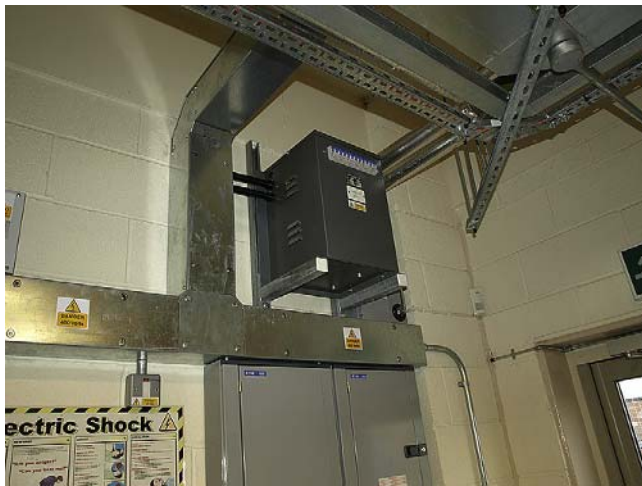
FIGURE 2.5 An isolating transformer supplying extra-low voltage socket outlets for use of portable tools in an industrial installation.
