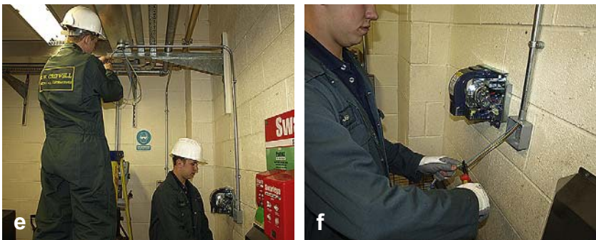
(e) Feeding should be done in such a manner as to prevent any cables crossing or becoming twisted. The operation needs care, and there must be synchronisation between the person feeding and the person who is pulling. The drawing-in can be assisted by using a cable-pulling lubricant. (f) After leaving some slack at the draw-in box, the cables can be cut to length (all M.W. Cripwell Ltd).
