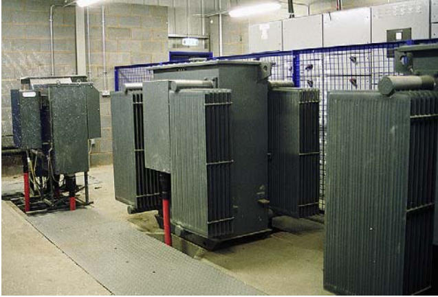
FIGURE 5.1 Main transformers in a factory building. Incoming supplies are from an 11kV ring main and feed two 800kVA, 11kV to 415V transformers. The distribution board in the sub-station use four-pole 1600A ACBs set at 1200A and a four-pole bus coupler rated at 2000A (W.T. Parker Ltd).
