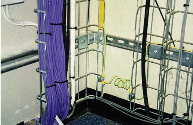
FIGURE 4.5 A commercial location where a cable riser is constructed from cable basket and carries cables for different types of circuits. Note the equipotential bonding conductors (W.T. Parker Ltd).
