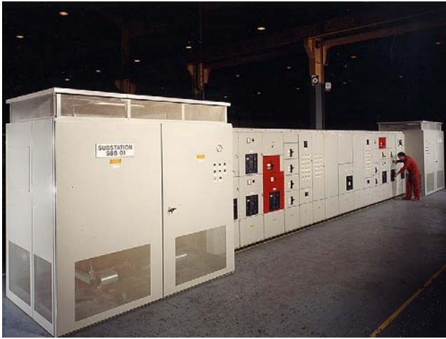
FIGURE 5.4 A sub-station comprising two 1600kVA, 11kV to 415V transformers, incoming and outgoing circuit breakers, fuseswitches controlling outgoing circuits and integral power factor correction (Durham Switchgear Ltd).
