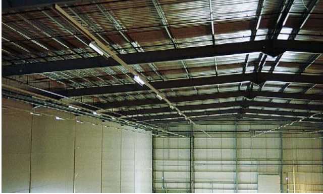
FIGURE 11.2 The busbar lighting units installed in a high-bay storage building. The lighting units have been installed and the installation is ready for the lids to be clipped on (W.T. Parker Ltd).
