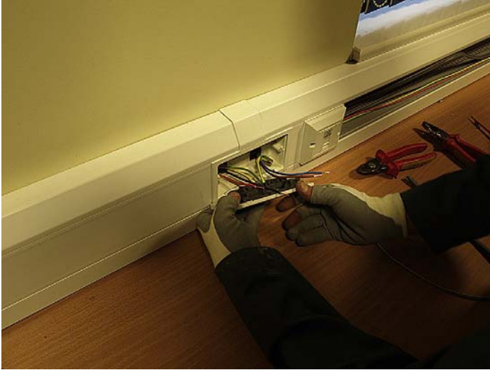
FIGURE 8.7 An extension to this installation will result in a mixture of colours from the old and current standards. A warning notice will need to be displayed (M.W. Cripwell Ltd).
