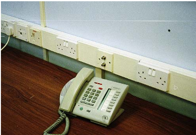
FIGURE 10.5 A typical office installation where data, telecommunication and power circuits are required (W.T. Parker Ltd).
