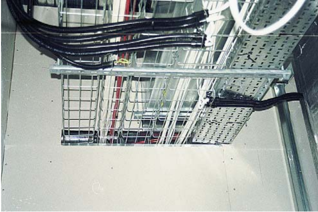
FIGURE 12.2 Cable runs fitted in the roof space above a suspended ceiling. Multi-compartment cable basket is provided, as well as cable tray for different circuit categories. Note the copex flexible conduits which carry feeds to specific locations (W.T. Parker Ltd).
