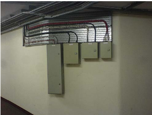
FIGURE 8.3 This neat installation shows cable tray with PVC and FP cable systems used to good advantage in a distribution area.
