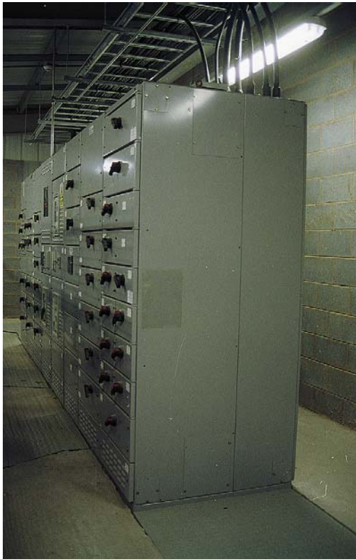
FIGURE 2.6 IEE Regulation 513 requires that every item of equipment be arranged so as to facilitate its operation, inspection and maintenance. This switchboard is installed in a room provided for the purpose, with access space both in front and behind the equipment. This situation will allow access for proper maintenance (W.T. Parker Ltd).
