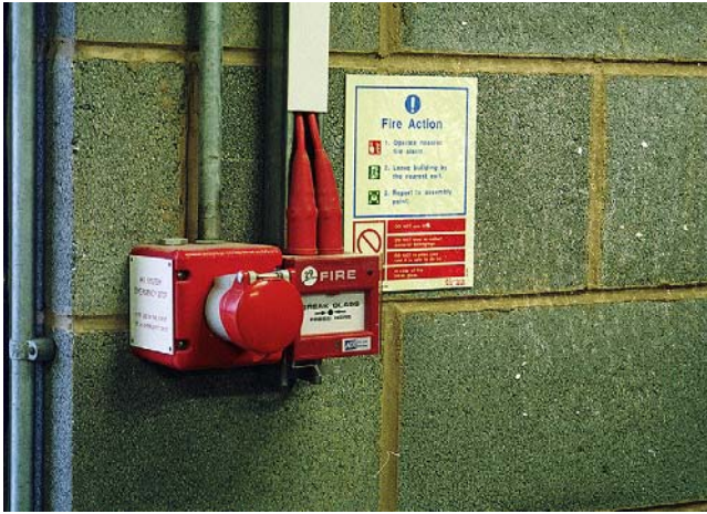
FIGURE 14.6 Emergency stop and fire alarm are grouped together in this industrial installation. MI cable in use to connect the break glass fire alarm control.
