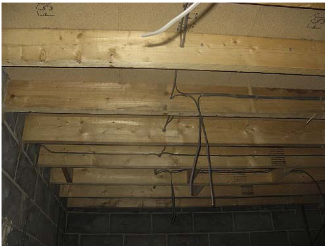
FIGURE 13.5 During building construction, it is possible to gain access to joists from either above or below. Here the upper floor has been laid but access for wiring is still possible from below. Joists have been bored and cable runs made prior to the ceiling being fitted (NBK Electrical).
