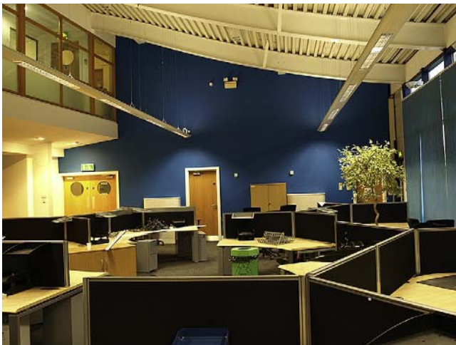
FIGURE 10.3 Office lighting fitted in integral trunking which houses the control units as well as the light fittings, the whole being suspended from the roof structure.
