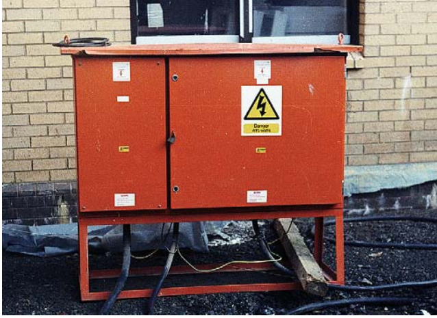
FIGURE 7.2 Load centre for a temporary installation on a construction site (William Steward & Co).
