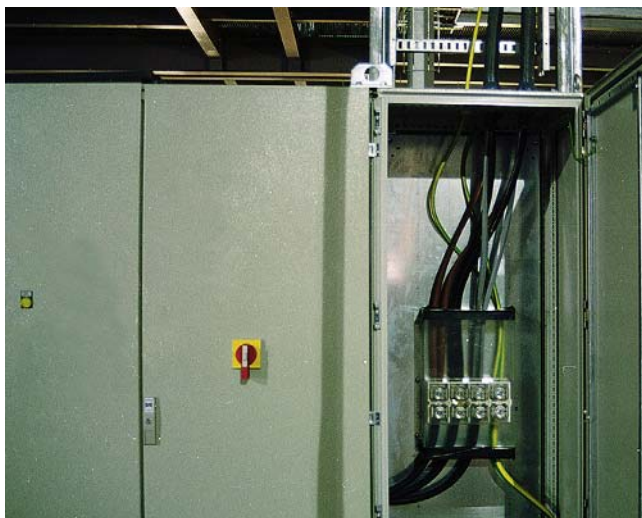
FIGURE 4.8 The use of cables connected in parallel ease the installation task and can often result in a more economical scheme. This view shows a distribution circuit employing parallel multi-core 415V cables, run on cable ladder, feeding a distribution board. The cables are 120mm 2 multi-core PVC insulated SWA copper. Had parallel cables not been used, 300mm 2 cable would have been needed (W.T. Parker Ltd).
