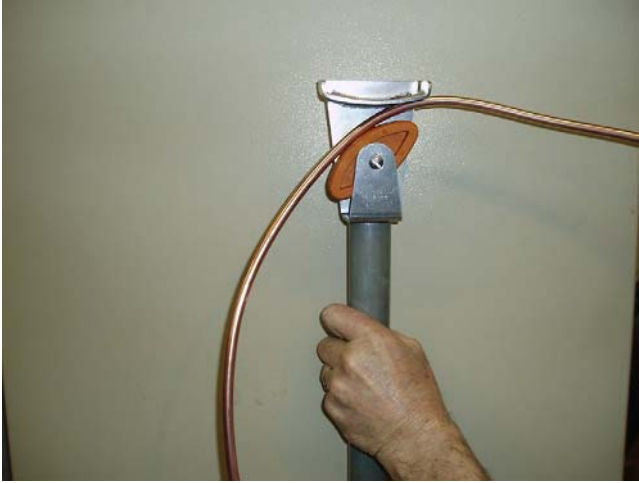
FIGURE 14.3 Bending and setting of MI cable. These operations can be more easily done by means of the simple tool illustrated (Wrexham Mineral Cables).
