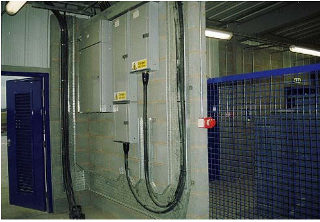
FIGURE 12.5 A neat installation of cable tray in a sub-station carrying feeds to individual distribution boards (W.T. Parker Ltd).
