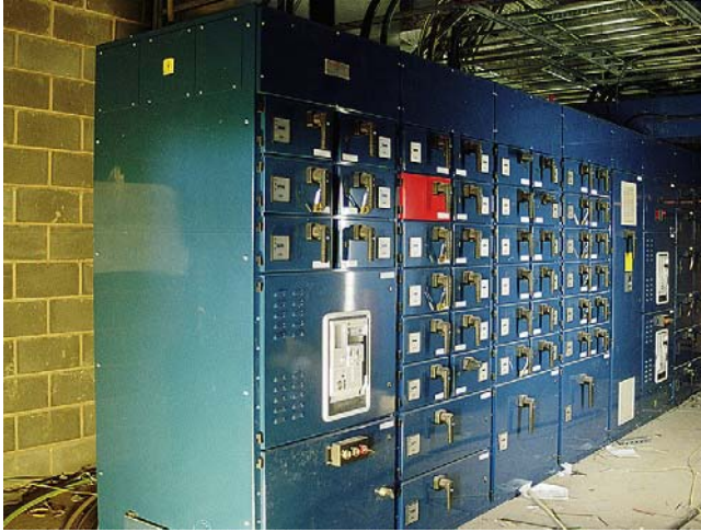
FIGURE 5.3 A switchboard for use in an industrial premises. The board incorporates over 60 outgoing switches as well as main ACBs, bus-section switches and metering facilities (Pandelco Ltd).
