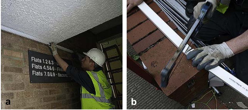
(a) The mini-trunking is offered up on site and marked to indicate the location of the bend. (b) Using a fine-tooth hacksaw, the conduit is cut at the back and on one side to suit the angle of bend required.
