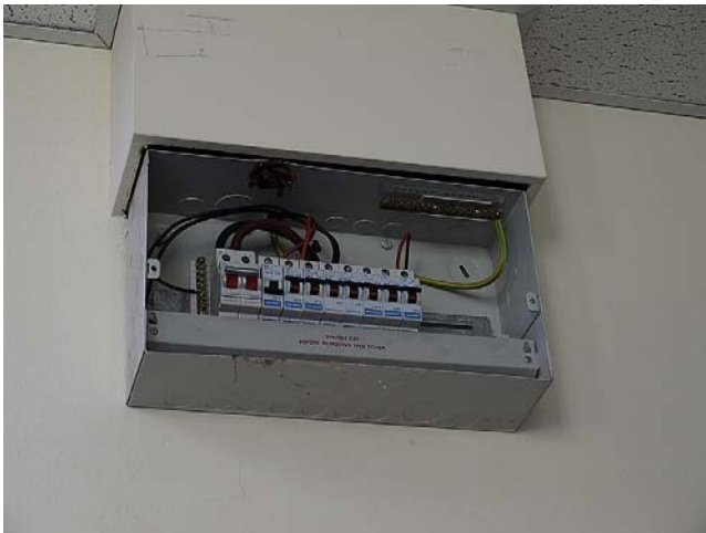
FIGURE 5.19 An eight-way metal-clad consumer unit with MCB protection.
