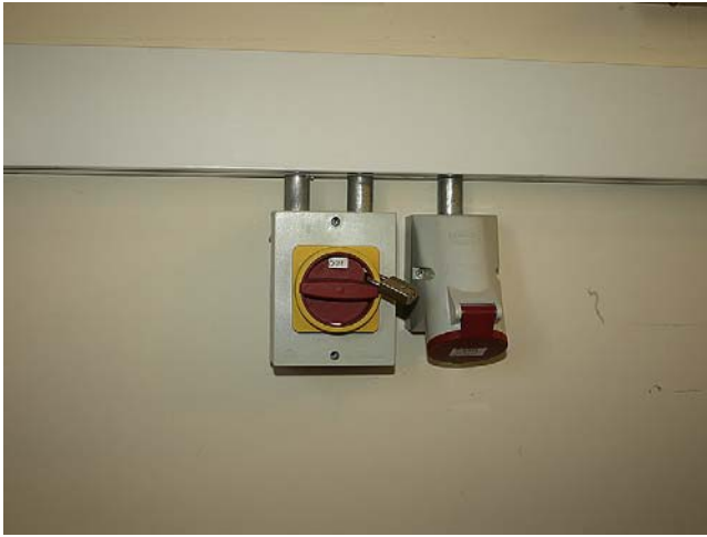
FIGURE 1.2 To comply with the Electricity at Work and IEE Regulations, it is necessary, in appropriate circumstances, to provide means to 'prevent any equipment from being inadvertently or unintentionally energised'. Isolators with provision for padlocking in the isolated position are available to meet this requirement (M.W. Cripwell Ltd).
