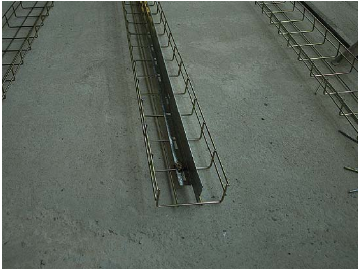
FIGURE 8.12 Segregation of circuits is a requirement of the Regulations. In this view, cable basket, ready for erection, has been fitted with a dividing barrier (M.W. Cripwell Ltd).
