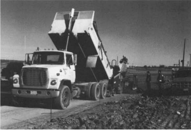
Figure 8.2 Dump truck used for the transportation of concrete during the construction of a roller-compacted concrete pavement.
