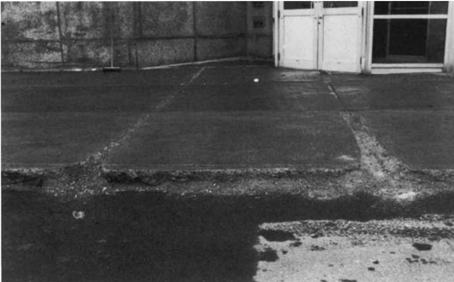
Figure 7.2 Frost damage on a part of a concrete structure with easy access to moisture.
