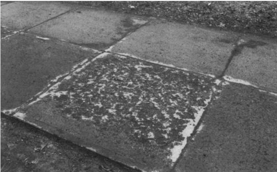
Figure 3.2 Severely scaled section of a sidewalk (due to freezing in the presence of de-icer salts) next to slightly damaged sections.
