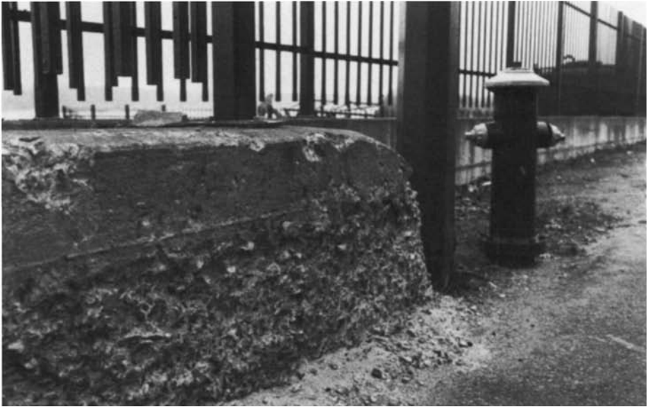
Figure 7.3 Concrete highway structure exposed to splashing of water containing de-icer salts.
