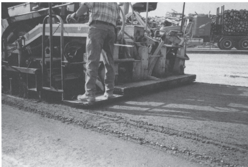
Fig. 18.12 The surface of the roller-compacted high-performance concrete just after the placing by the asphalt paver.
