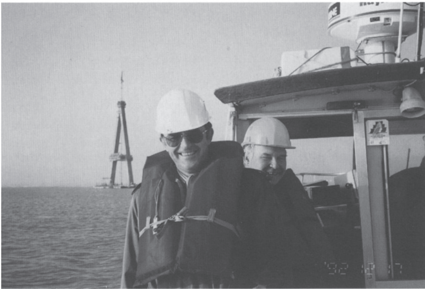
Fig. 4.15 'Pont de Normandie' under construction. One of the two pylons in construction during a visit of the author (pale hat) in December 1992 with Jean-François de Champs (darker hat) of Campenon Bernard Company.
