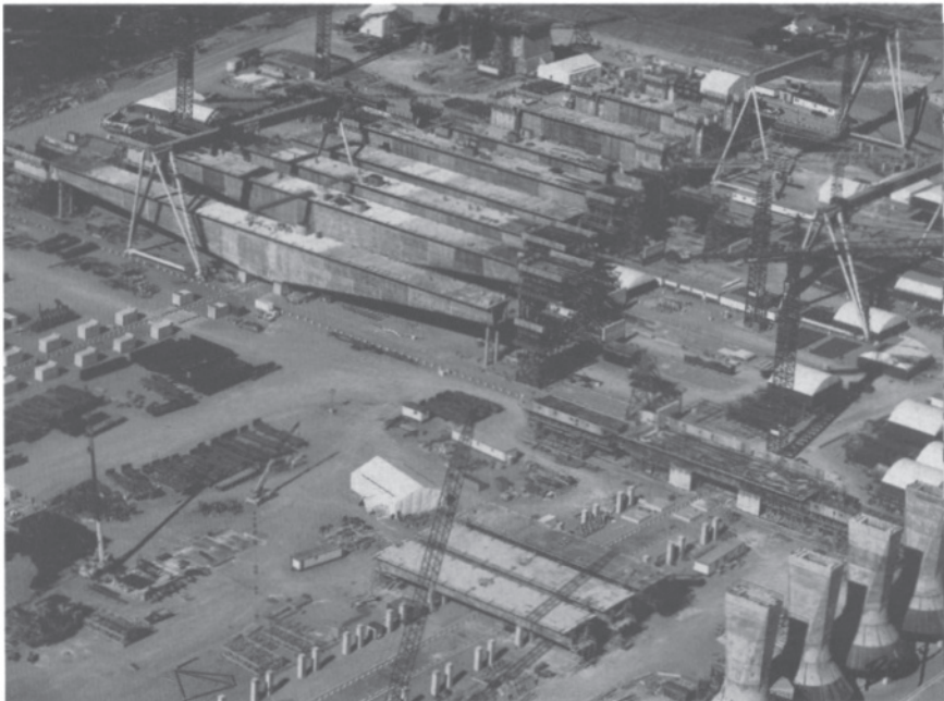
Fig. 4.23 Assembly yard (Prince Edward Island side) for the Northumberland Strait Crossing Fixed Link. Courtesy of G.Tadros.
