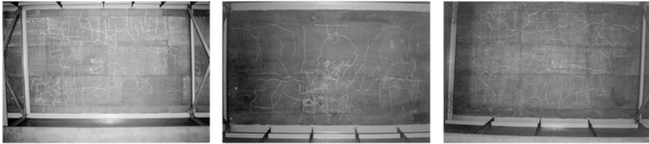
(b) Images of damage level II
