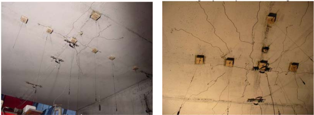
(a) At load level of 100 kips
