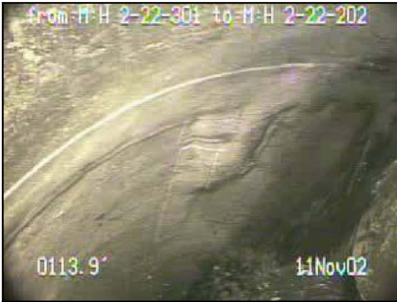
Figure 4. Blister in liner
