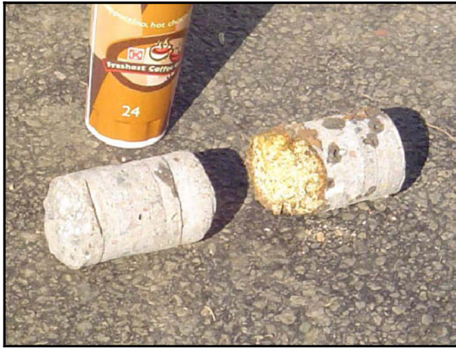
Figure 9. Core samples from 750 mm concrete pipe section
