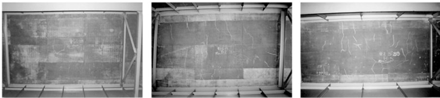
(c) Images of damage level III
