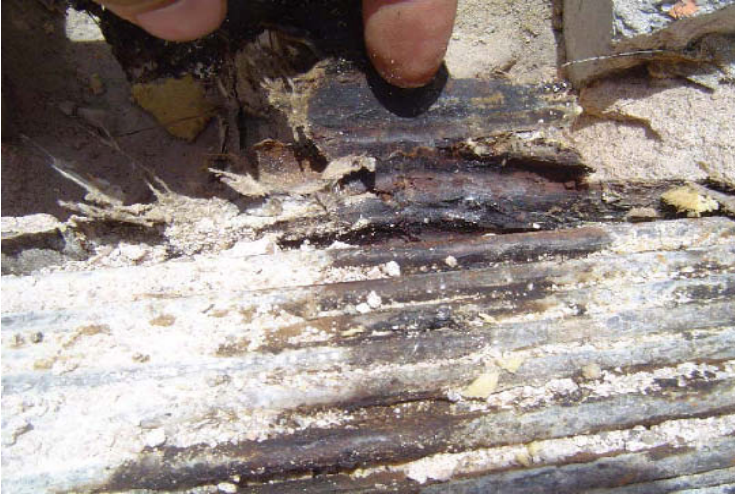
Figure 7. Typical condition of prestressing wires.
