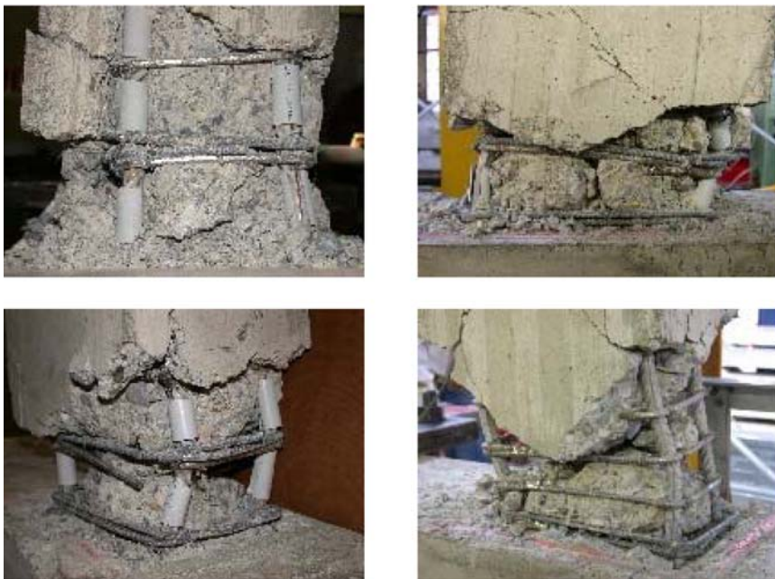
Fig. 17. Details of the plastic hinge at the final stage.
