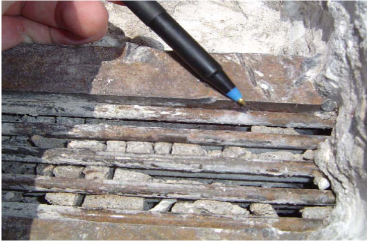
Figure 9. Typical condition of exposed anchorage.
