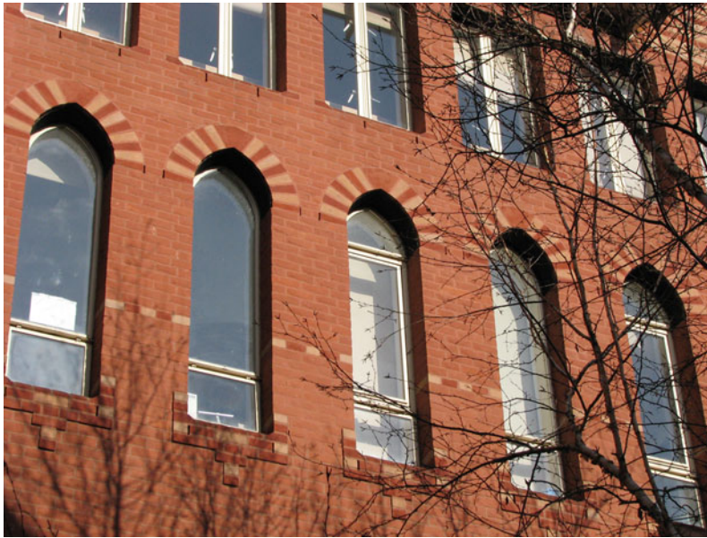
Daylight, Indoor Illumination, and Human Behavior. Figure 10 High-level glazing and deep window reveals
