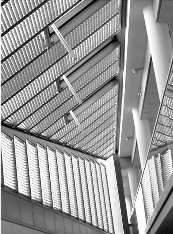
Daylighting Controls, Performance and Global Impacts. Photo 23
