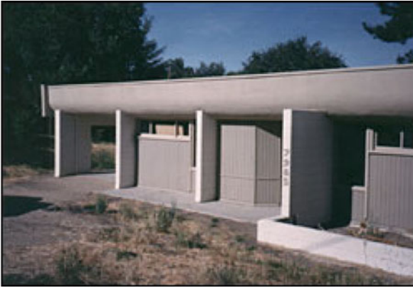
Passive Solar Heating in Built Environment. Figure 16 A mass roof: the Skytherm house in Atascadero California by Harold Hay (photo source: Evelyn and Harold Hay Fund at Cal Poly, San Luis Obispo, USA)
