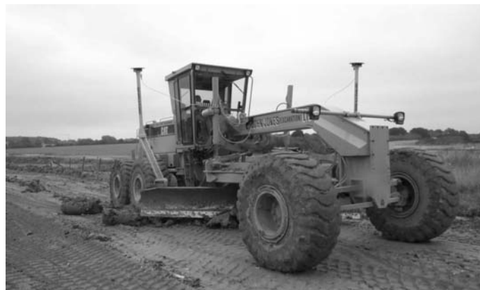
Figure 11.93 • Dual GNSS antennas mounted at each end of a grader blade (courtesy Trimble & KOREC Group).
