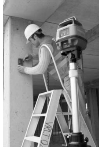
Figure 11.85 • Using a laser sensor to define a level line on a column (courtesy Pentax Industrial Instruments Co Ltd).
