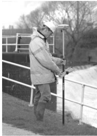
GNSS equipment on site
