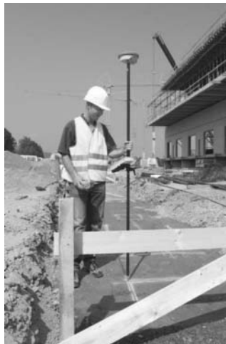
Figure 11.30 • Setting out using a GNSS rover – it is important to keep the pole vertical and still (courtesy Leica Geosystems).
