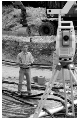
Figure 11.27 • One-person setting out using a Leica remote control unit on a pole-mounted 360° reflector working with a 1200 series robotic total station (courtesy Leica Geosystems).
