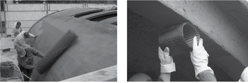
Figure 1.6 Repair and retrofitting with TRC by applying an external layer of TRC on concrete components. (From Lieboldt, M. and Mechtcherine, V., Cement Concr. Res. , 52, 53, 2013.)
