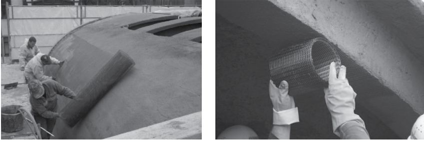
Figure 3.8 Strengthening of a barrel-shaped roof made of reinforced concrete by a layer of TRC. (From Lieboldt, M. and Mechtcherine, V., Cement Concr. Res. , 52, 53, 2013.)
