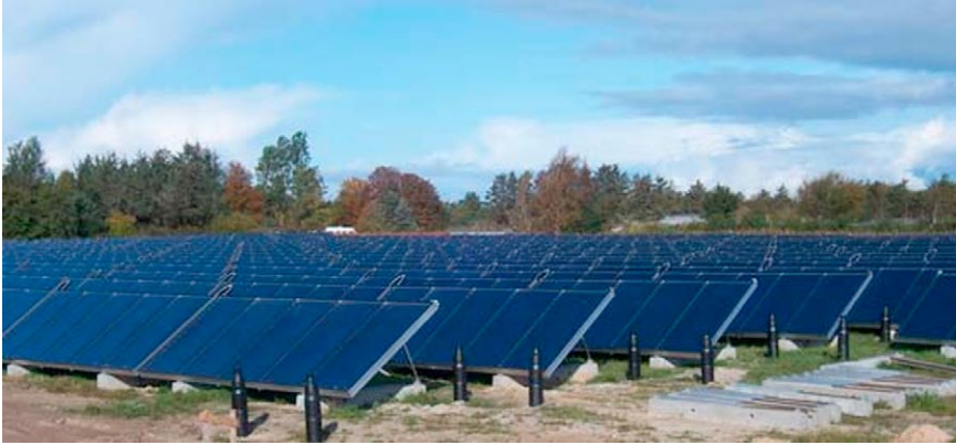
Figure 14.8 Array of solar collectors in Strandby.
