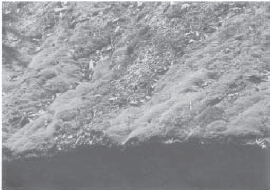
Fig 2.17 Decaying thatched reed on the roof of the Outer Tamagaki Gateway, Inner Shrine, Ise (1991 photo- graph of 1965–73 building)
