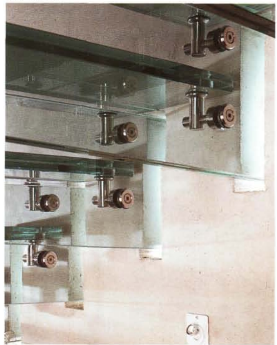
Fig. 7.8 The glass cantilevers in the staircase at the Pilkington Exhibition Centre, Lathom (courtesy of Pilkington/Chris Gascoigne)
