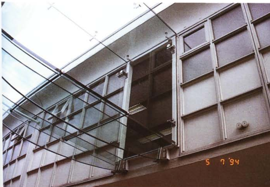
Fig. 7.7 The glass beams that support the glass footbridge between 2 offices of Kraaijvanger•Urbis in Rotterdam (courtesy abt)
