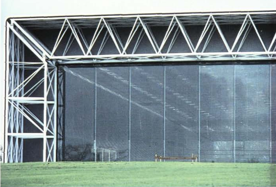
Fig. 7.11 Sainsbury Centre for the Visual Arts glass fins (courtesy of Foster and Partners)
