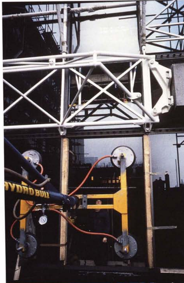
Fig. 17.1 Mechanical handling on site of a large pane of glass (courtesy of M. Elkan Photo)
