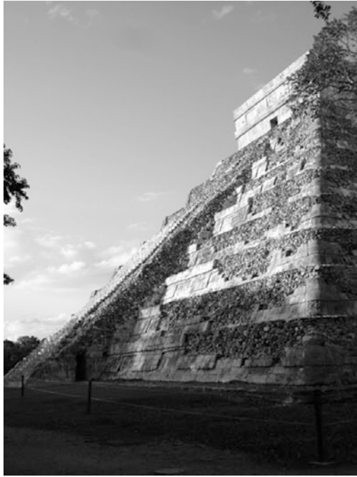
Fig. 10. The southwest stairway of the pyramid of Kukulcán in precarious conditions. Photograph by the author
