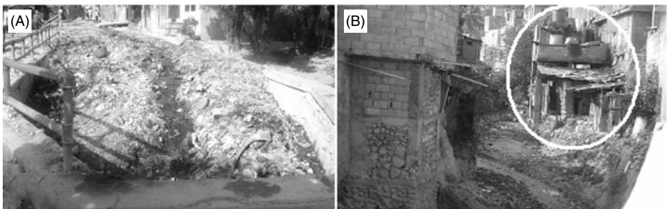
Figure 8.4 Typical flooding and pollution problem in Port-au-Prince: (A) solid wastes and sediments disposal into open channel; (B) anarchic building on floodplains of natural storm drainage channel.
