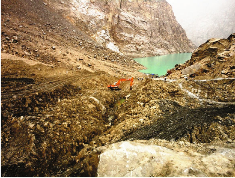
Fig. 1.24 Excavation of spillway in the debris of the Attabad rockslide dam, Hunza valley, northern Pakistan. The Hunza rockslide dammed lake is visible in the background. Photograph taken on April 18 (Day 102 of impoundment) when the lake level was at about 2,405 m a.s.l., 30 m below the eventual overflow elevation ( Pamir Times photograph)
