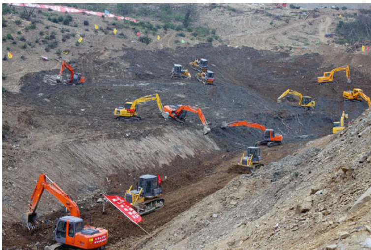
Fig. 10.11 The Tangjiashan sluiceway under construction (Provided by Water Resources Bureau of Mianyang city)
