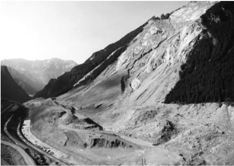
Fig. 2.11 Looking downstream across the 1987 Mount Zandila rock slide–rock avalanche and the Val Pola landslide dam. An open-channel spillway is under construction across the landslide dam. A twin-bore diversion tunnel (Fig. 2.13) passes through the granite bedrock valley wall on the lower left
