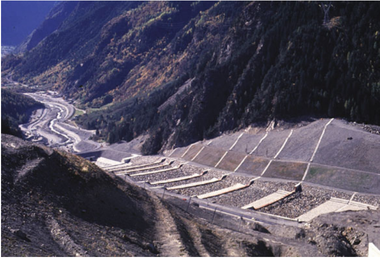
Fig. 2.12 Open-channel spillway, concrete sills, and a check dam under construction on the downstream slope of the Val Pola landslide dam
