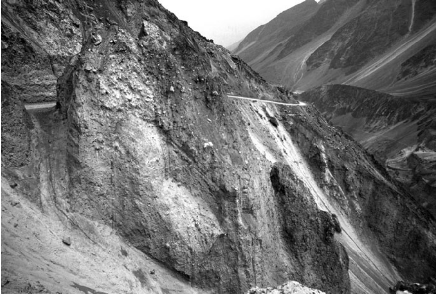
Fig. 6.11 Mountain road cut through a rock avalanche, the Bilchar event, in Bagrot valley, Gilgit District. The vertical cuts testify to the strength and compaction of the rock avalanche material, but rainfall and snowmelt can generate sudden collapses or debris flows at the surface. The landslide once formed a dam on the Bagrot River [28]
