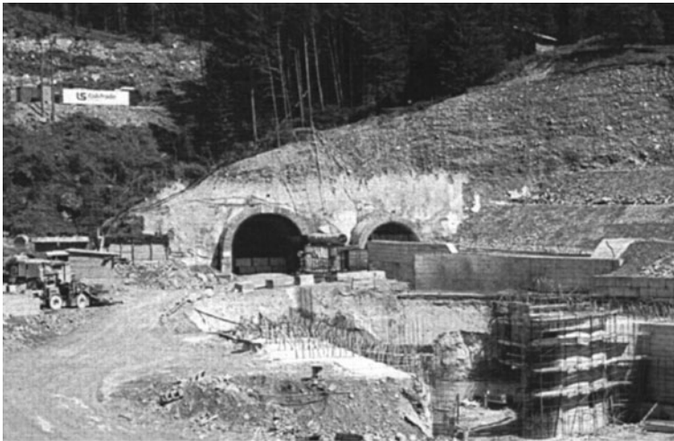
Fig. 2.13 Exit portals for the twin-bore diversion tunnel that carries the Adda River around the Val Pola landslide dam. The tunnel on the right was operational at the time of the photo, and the left-hand tunnel was near completion
