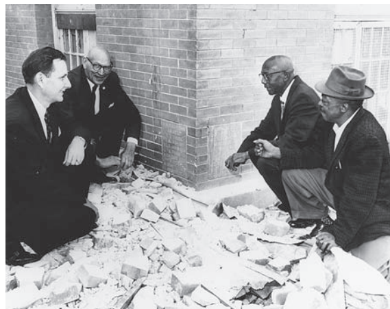
City officials and African American civic leaders inspect the cornerstone of the Colored Carnegie Library during its demolition in 1962. (RG A13-2144, Courtesy HMRC, Houston Public Library.)
