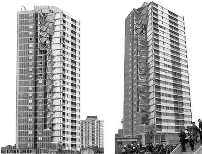
FIGURE 9.1 Damage at Ronan Point apartment building.
