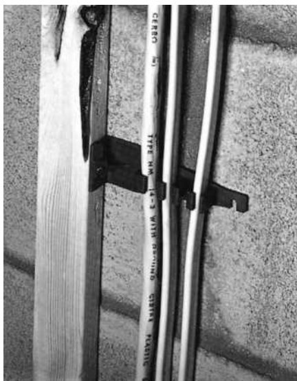
FIGURE 4-29 Devices that can be used to meet the Code requirement to maintain a 1¼ in. (32 mm) clearance from framing members.
