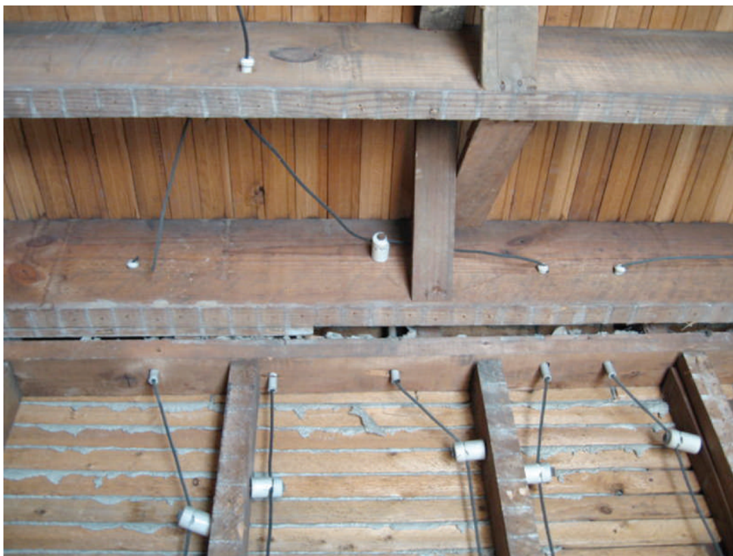
FIGURE 4-6 Photograph of a typical knob-and-tube wiring from the 1930s.
