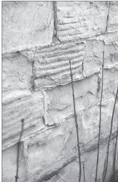
Figure 4.25 Face bedded masonry wall. The outer layers of the stone can easily be ‘peeled’ away by the action of salts and frost. In this photograph the stones that have deteriorated the most are face bedded.
