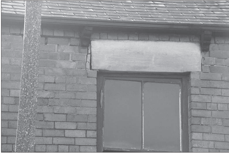
Figure 4.3 Distorted window opening in a damaged building. The top sash has been regularly adjusted so that it will close. What will the carpenter do when she gets down to the glass?
