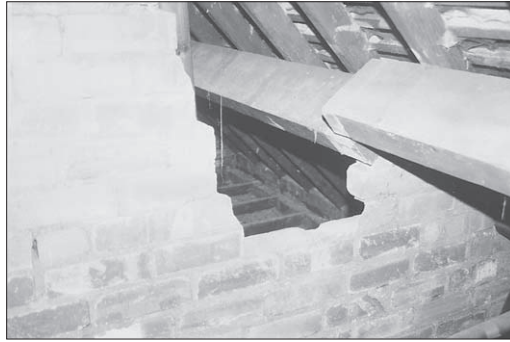
Figure 7.5 Inadequate support to purlins at the end bearing. These purlins are poorly supported by this partial party wall.
