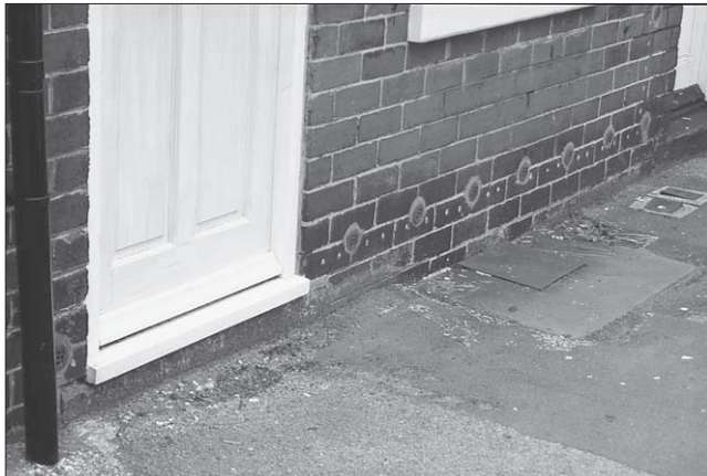
Figure 5.11 This photograph shows ceramic ‘drying tubes’ that have been installed in a brick wall. The smaller filled holes close by suggests that a chemical damp proof course may also have been installed.
