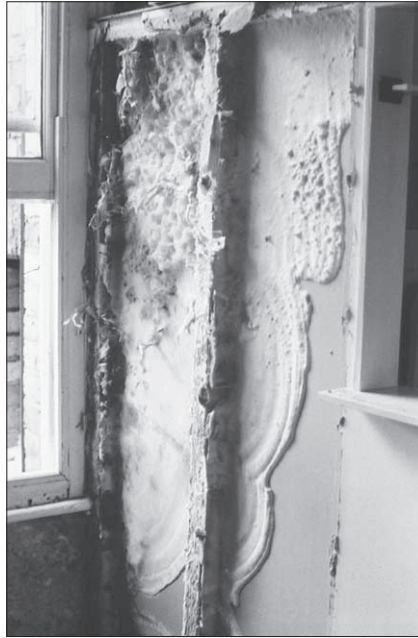
Figure 6.1 Photograph of dry rot within a timber partition. The plasterboard to the wall has been removed to reveal a luxurious dry rot growth. The outbreak began in the vertical timber stud that is fixed to the inside face of the external wall (to the LHS of the picture). The source of moisture and the cause of the outbreak was a leaking gutter that saturated the wall.
