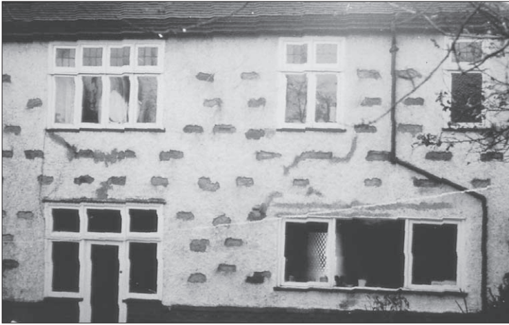
Figure 4.18 A dwelling that has had its cavity wall ties replaced. The technique probably involved the complete removal of the defective wall ties. The guarantee for this work would have to be checked and should be backed by an appropriate insurance scheme.
