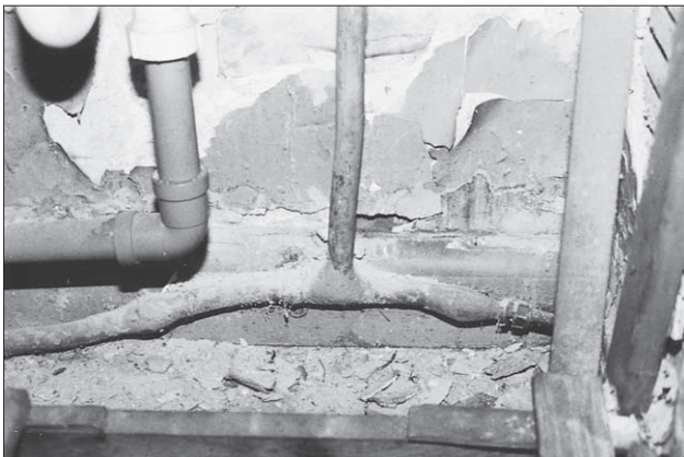
Figure 10.2 Lead water pipes are clearly thicker than other types. The bulbous joints shown in this photograph are typical of this material.
