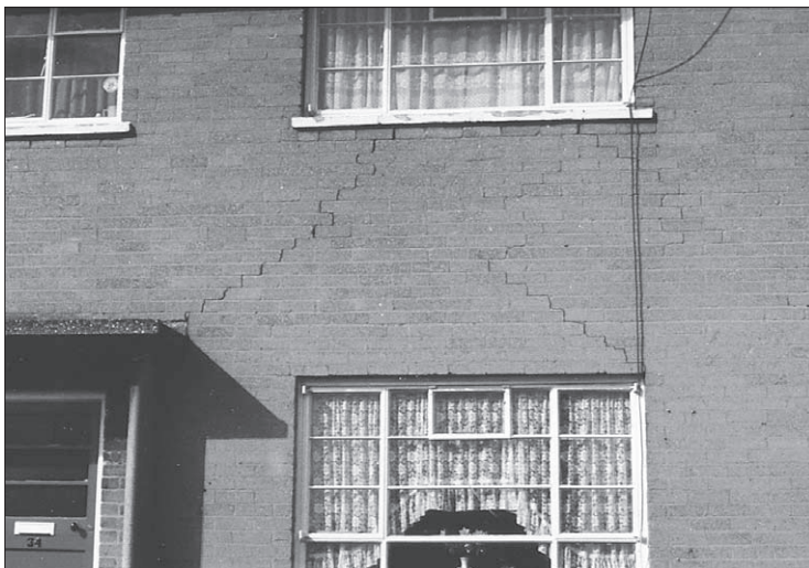
Figure 4.21 Cracking to a masonry elevation caused by expansion of brickwork. These semi-detached properties are built of calcium silicate bricks that are vulnerable to expansion defects.
