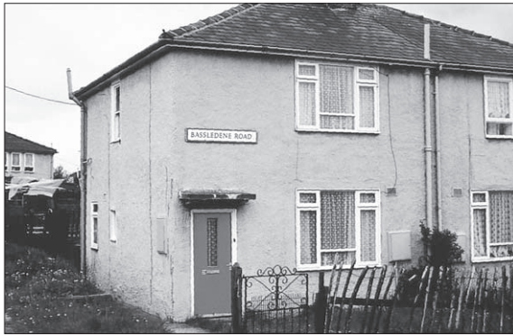
Figure 12.4 Boot house. The externally-rendered exterior can make them difficult to identify. Vertical cracking at the corners is a very common feature.
