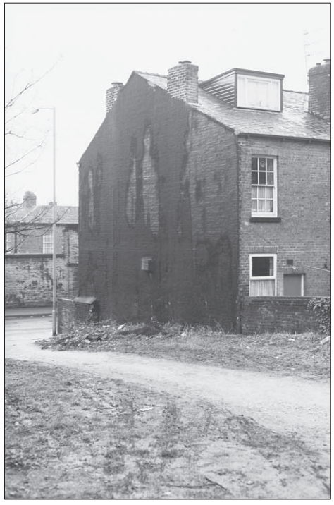
Figure 5.5 A gable elevation of a house that has been treated with a bitumen-based compound in an attempt to improve its moisture resisting properties.
