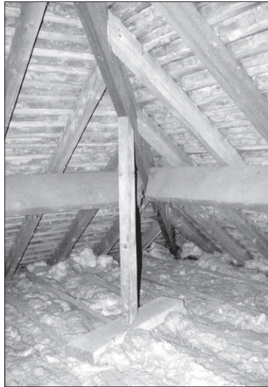
Figure 7.8 The hip rafter to this roof was deflecting because the wall plates were being spread apart by the thrust of the roof slopes. There were no dragon ties to restrain them. A builder had inserted a crude vertical strut to take the weight of the hip rafter. This was supported off the top of the ceiling joists below. A clearly inadequate solution.
