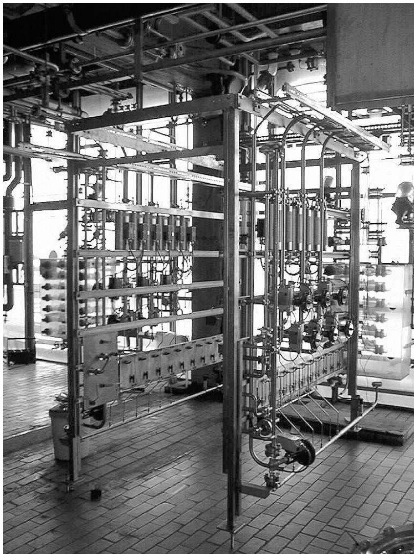
Fig. 14.7 Production plant for the synthesis of a metal-organic chemical using minimixers (Merck, Darmstadt, Germany).
