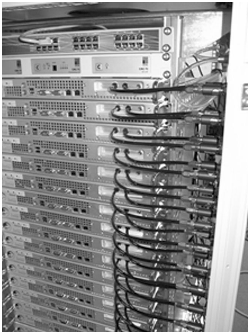
Fig. 14.13 Liquid-cooled server cluster (Atotech, Berlin, Germany).
